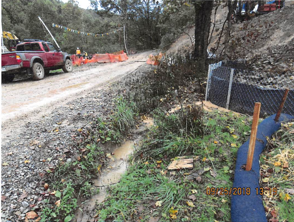
Photo 5: Sediment laden water entering UNT of Knowls Creek near station 3634+00 from failed perimeter controls.
