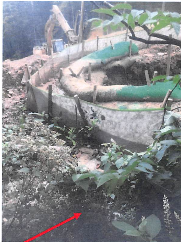
BMP near Station #9911+00 being overwhelmed and sediment flowing under and through control. Arrow depicts where sediment laden water was leaving BMP.
