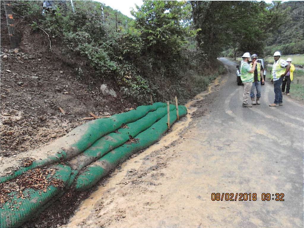
In process of stabilizing slope. Mud on road from crews performing maintenance.
