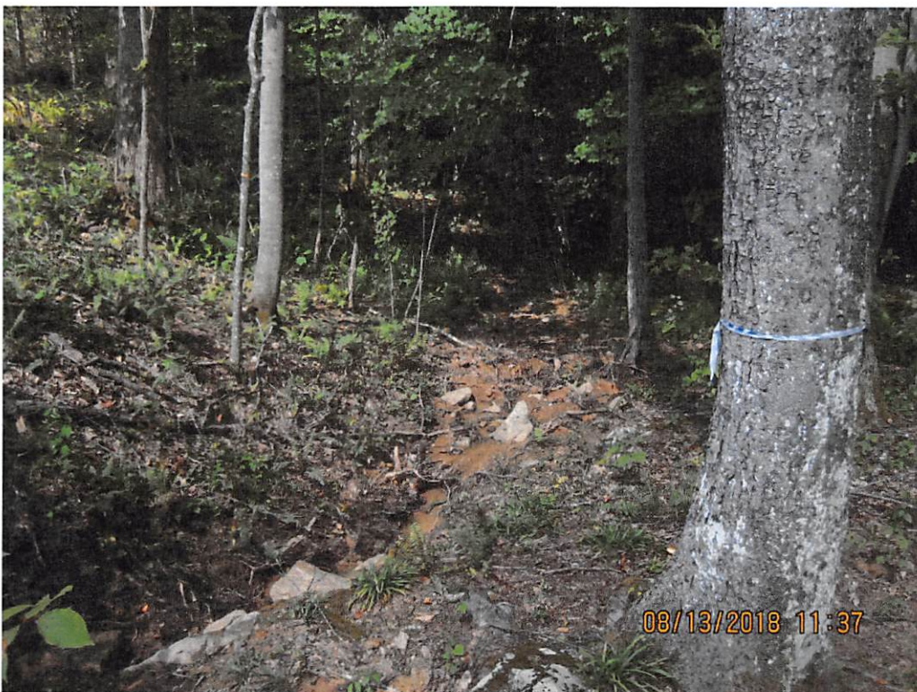
At St. 00+220 a series of perimeter controls used in a concentrated flow area had failed allowing sediment laden water to leave the site. Sediment deposits were noted in receiving stream A-104 creating Conditions Not Allowable in the Waters of the State.
