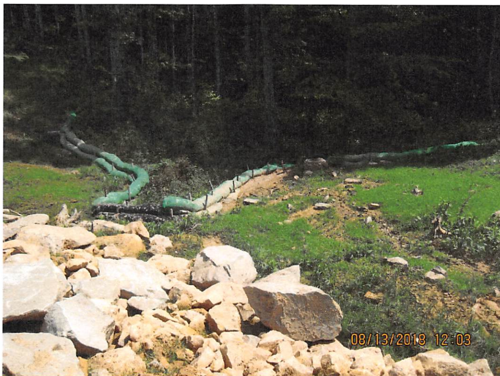
Maintenance needed for CFS below the east wall.
