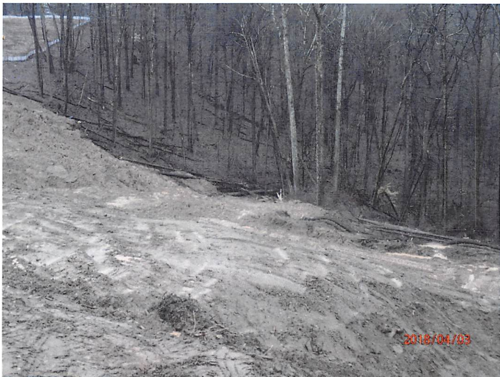
Slope above slip area.
