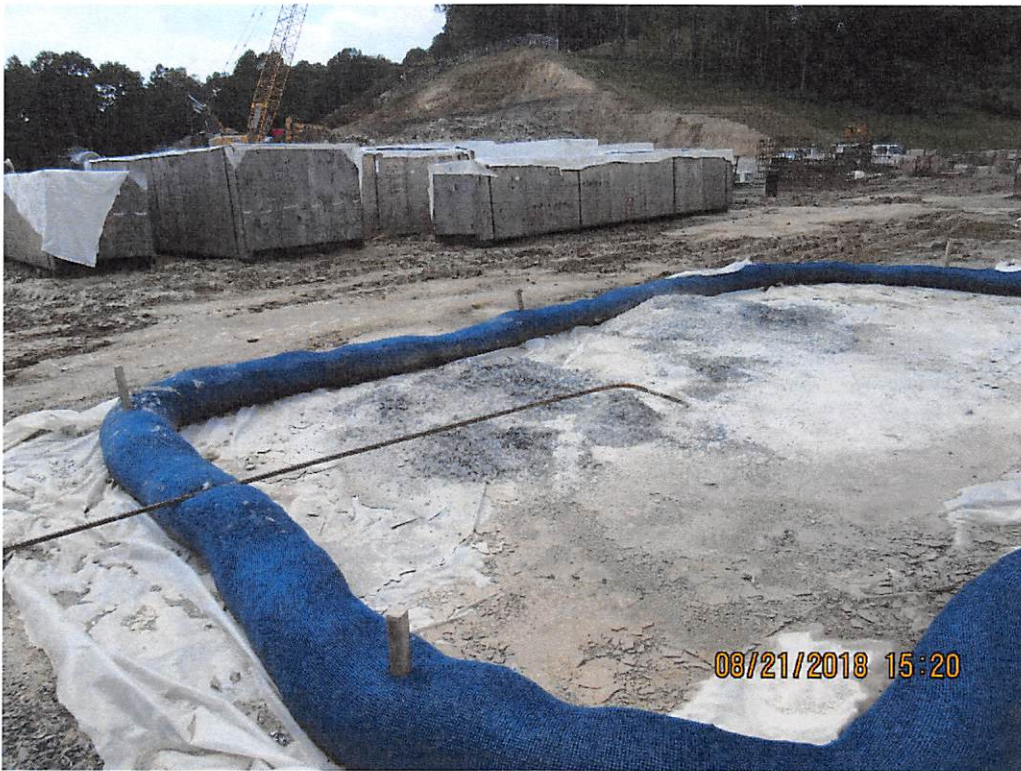
Photo 8: Improperly implemented control for concrete wash out area.
