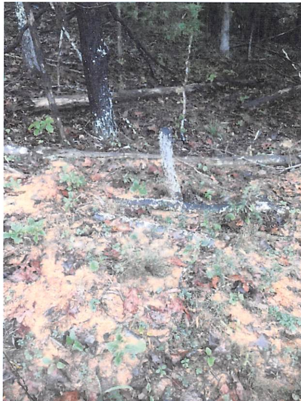
Off-site sediment deposits near station number 9779+00.
