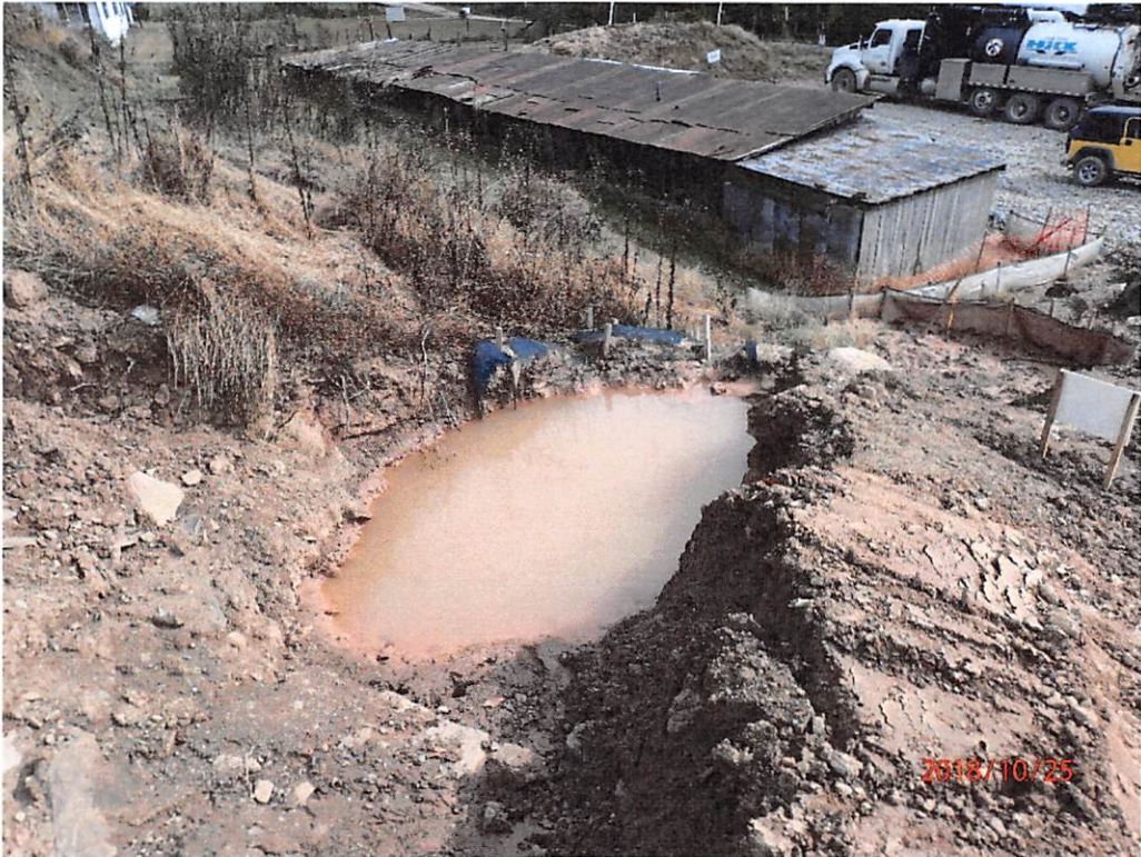
Overwhelmed sump near Sams Run.
