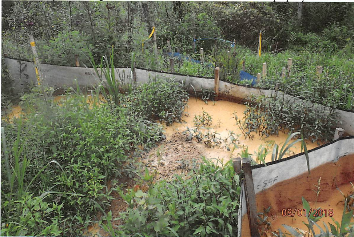
Perimeter controls adjacent to Goose Run that are overwhelmed due to improperly installed water bars. Both pictures show BMPs that are being undermined and overwhelmed due to excessive flow that is caused by improperly installed water bars.
