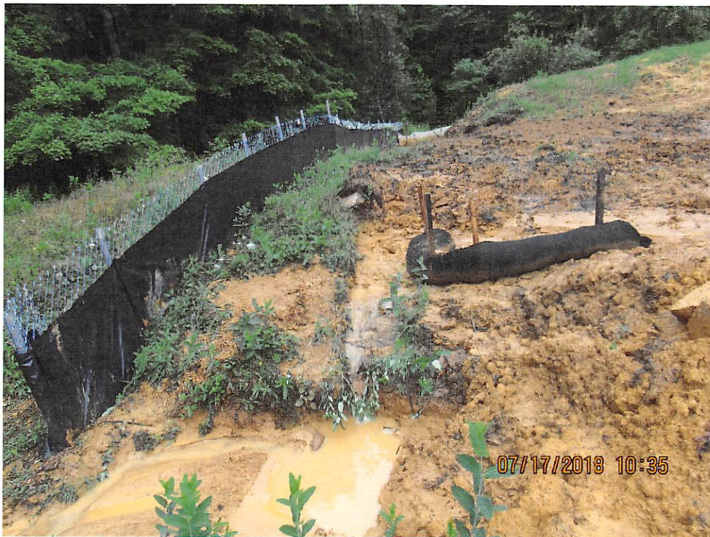
Photo 4: Station 5518+00 where water went around and undercut compost filter sock allowing sediment laden water to leave the site.
