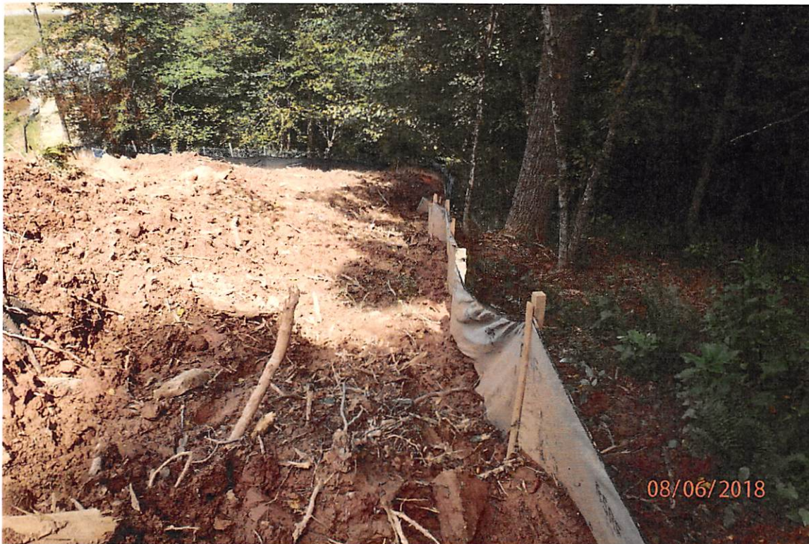
Concentrated flow being directed over fill slope into a sheet flow super silt fence from improperly installed water bars in Grass Run.
