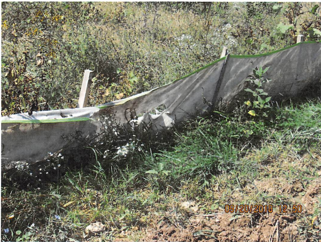
Photo 2: Silt fence needs replaced along access road 231.01 off Painters Run Road near station 10270+49.
