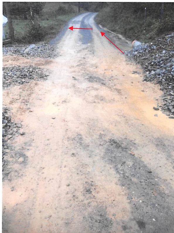
Sediment laden water flowing through culverted stream crossing and under road through culvert and into stream on other side of Ellison ridge road. Mud also present on road.
