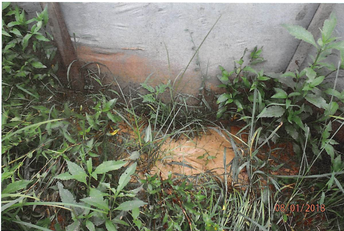
Perimeter controls adjacent to Goose Run that are undermined and allowing sediment laden water to leave the site.
