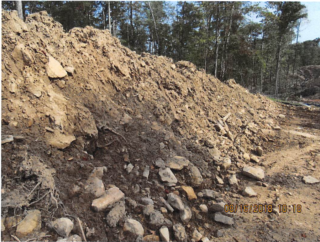
Photo 19: Northern view of waste pile with inadequate stabilization. (Photo taken near Bingham Road station 7450+00)
