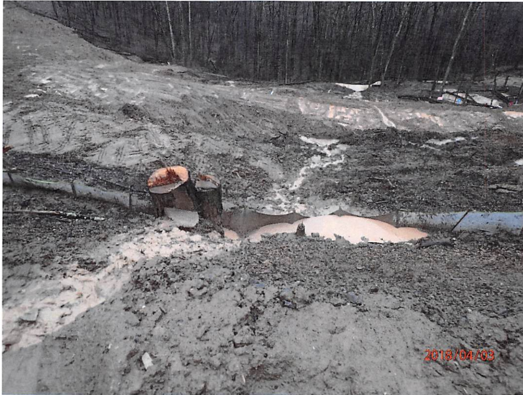
Concentrated flow eroding slope near slip.
