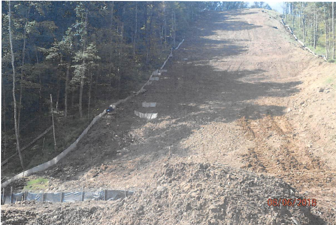
Improperly installed water bars and associated fill slope erosion in the Tenmile Creek watershed.
