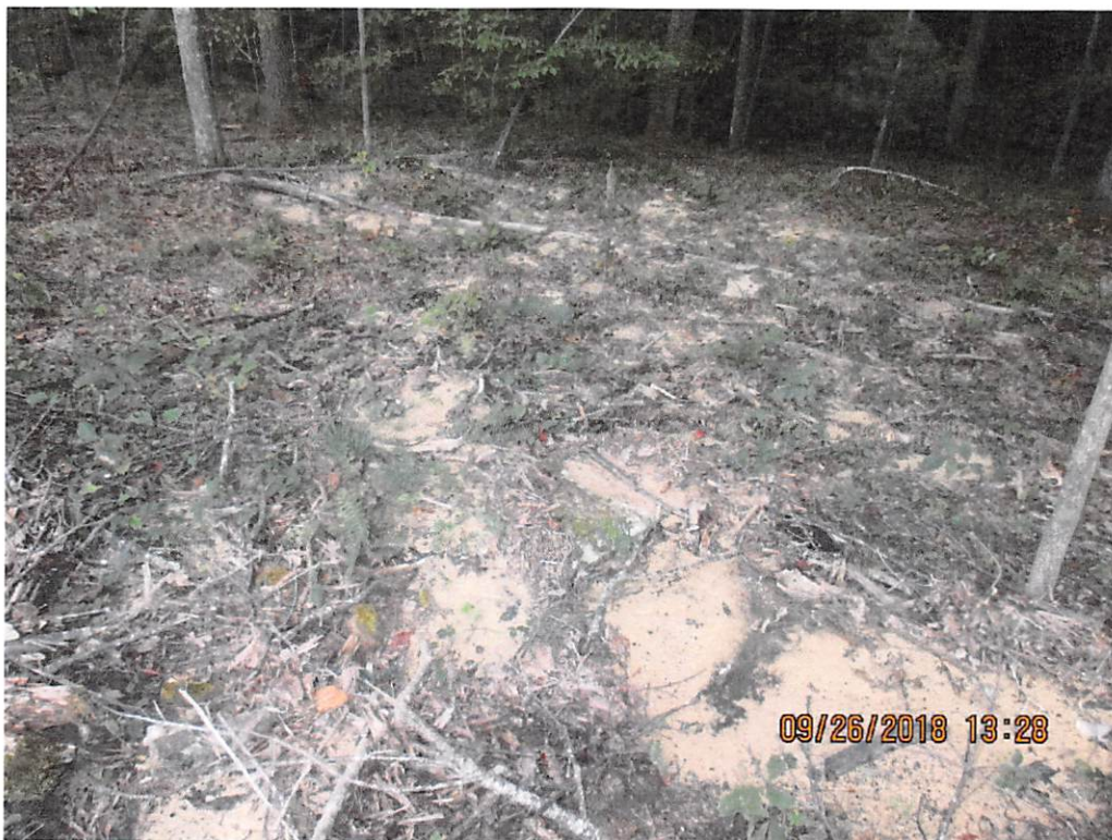
Off site sediment deposits located past LOD and being transported towards Streams S-H58 and TTWV-S-E58 near Station number 9899+00.
