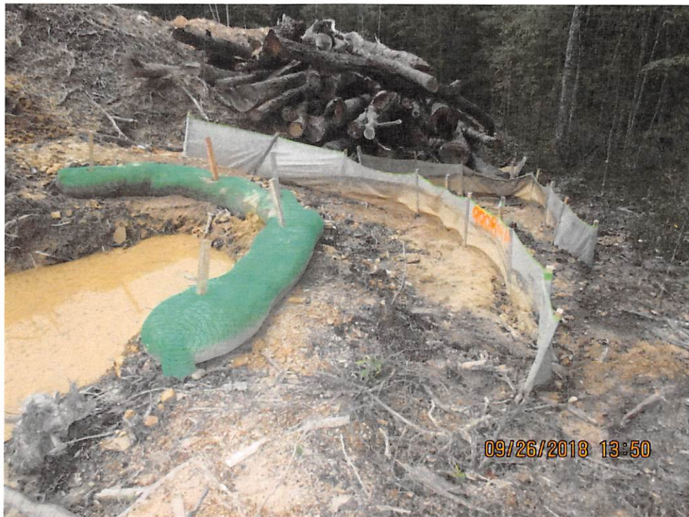
BMP at Station number 9908+00 being overwhelmed where off-site sediment deposits were present past the LOD.
