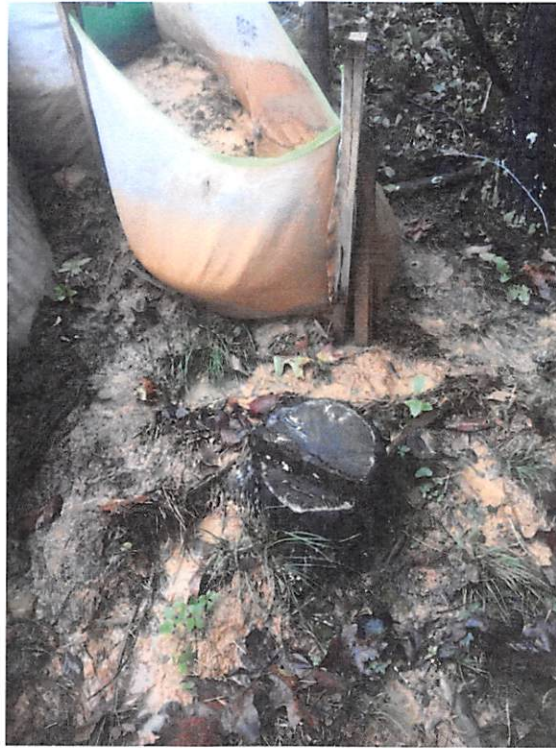
ROW near station numbers 9779+00 and 9778+00 where water bar outlets were being overwhelmed and sediment laden water was passing through and under and being transported past LOD.
