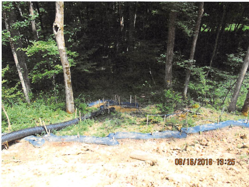
Photo 34: Recommended to lengthen 'J' hooks at end of pipe slope drains at station 6978+70.
