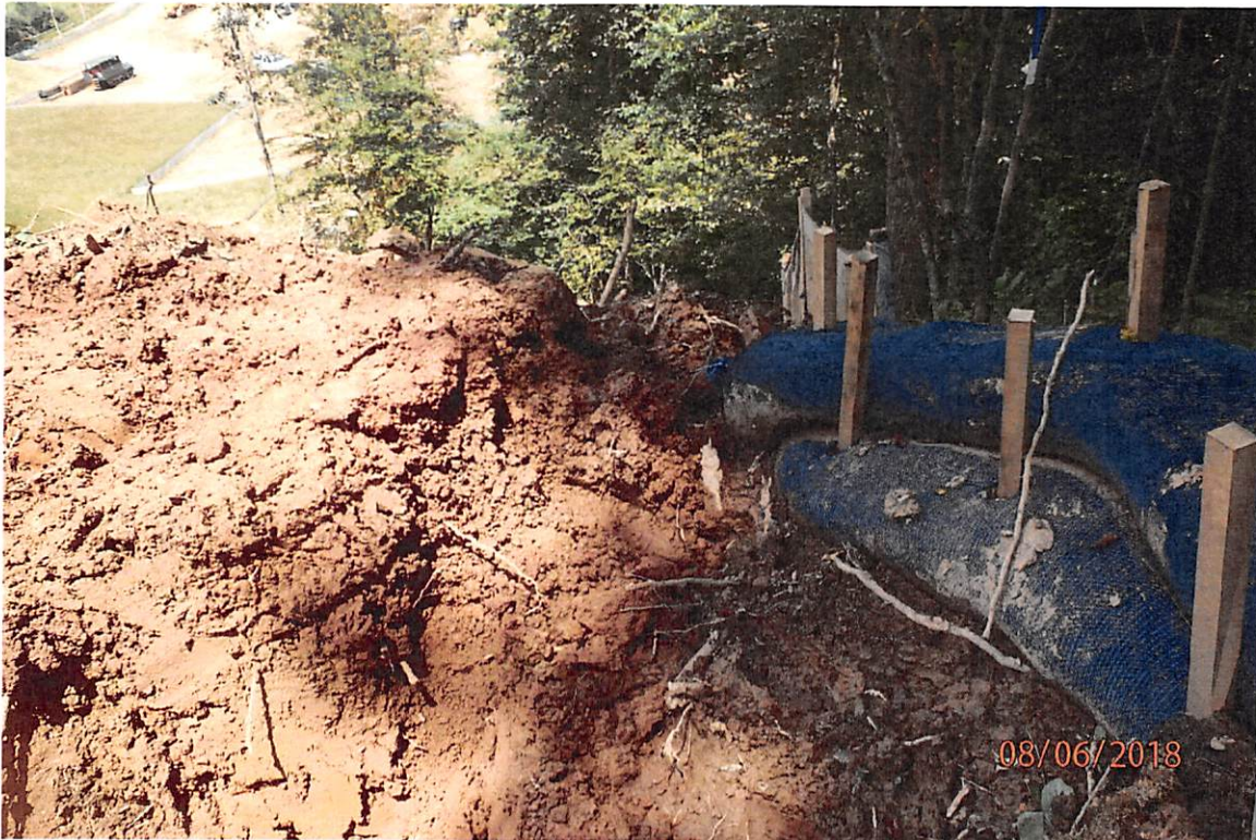
Water bar in Grass Run watershed that is improperly installed and led to CNA deposits in the stream.
