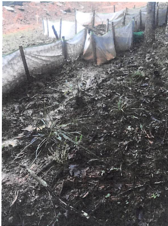
ROW near station numbers 9779+00 and 9778+00 where water bar outlets were being overwhelmed and sediment laden water was passing through and under and being transported past LOD.
