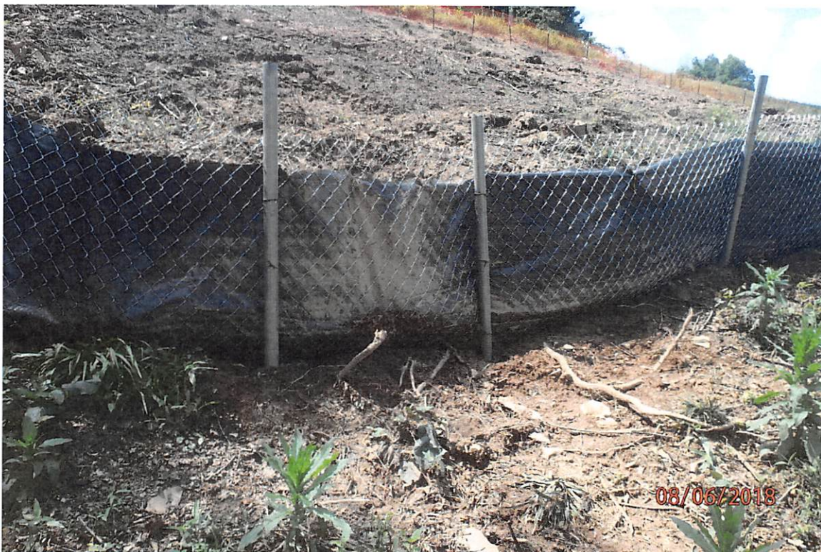
Perimeter control that was overwhelmed by concentrated flow and caused CNA deposits in Seal Run.
