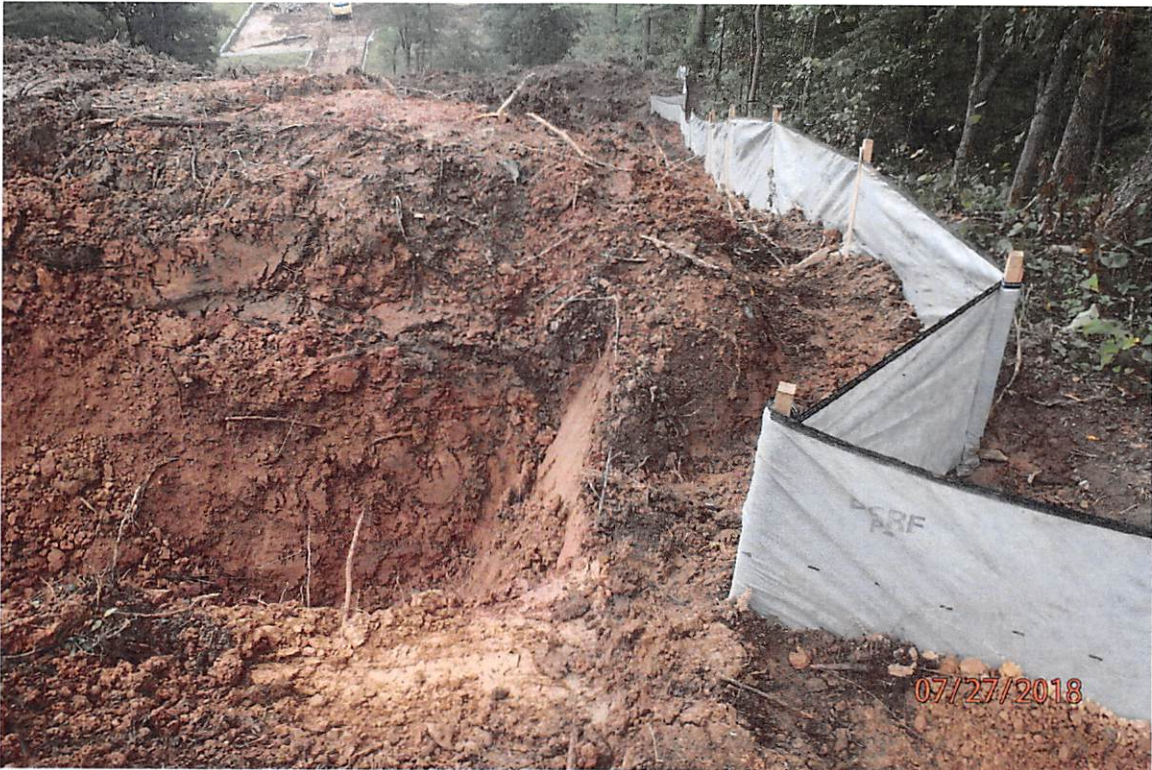
Improperly installed water bars that do not shed stormwater off site as designed.
