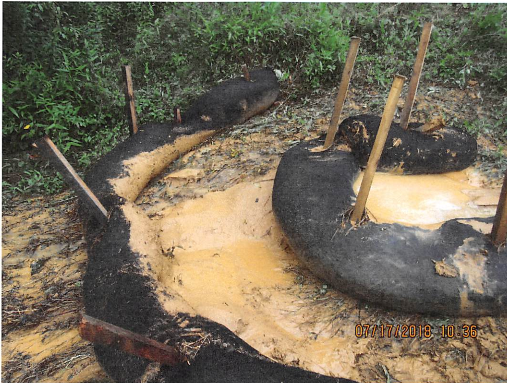
Photo 5: Next set of compost filter sock in sequence which was overtopped allowing sediment laden water to leave site.
