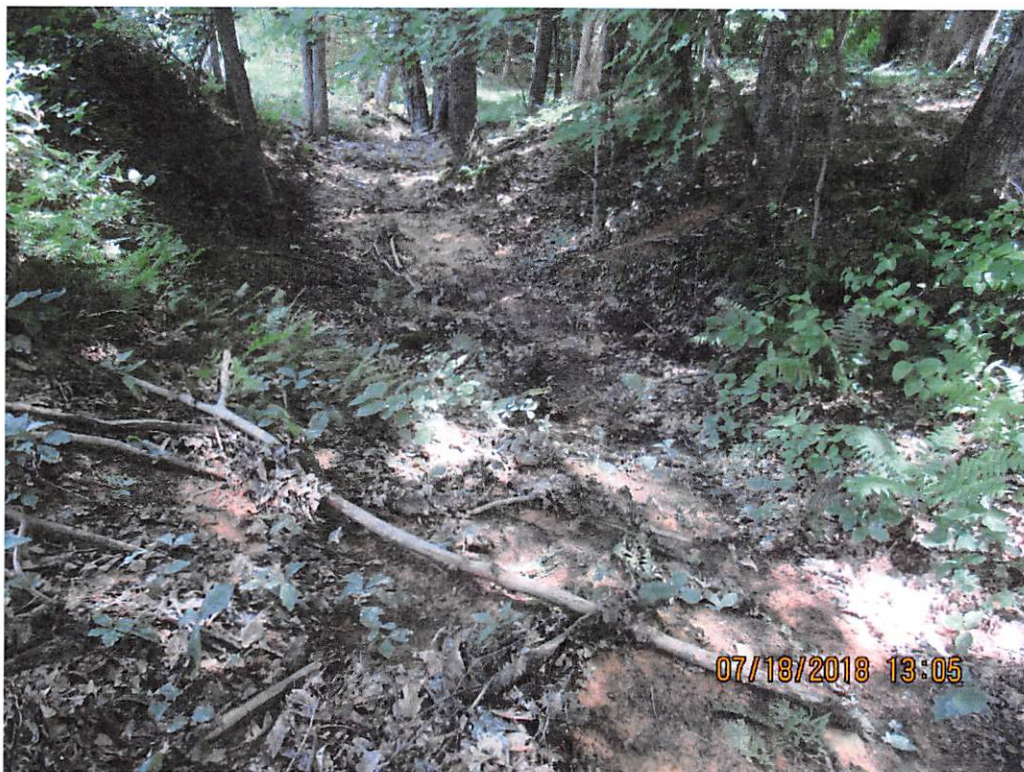
Photo 16: Down gradient view of scour from control failure at 6785+50.
