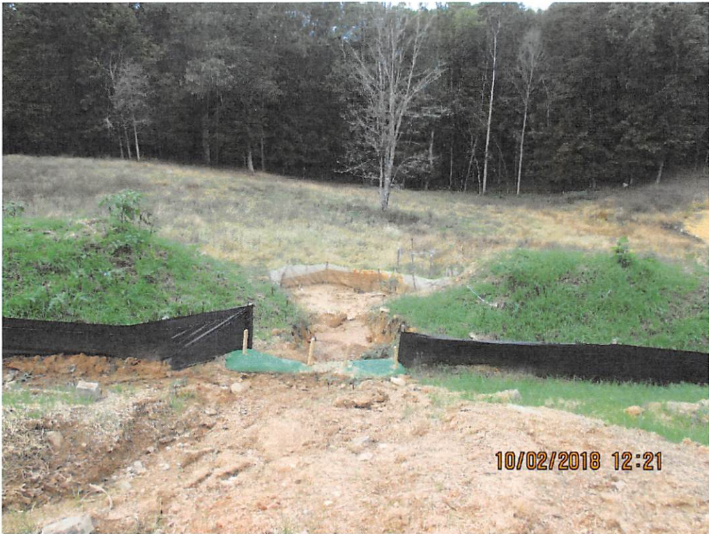
ROW near station #9687 where BMP is failing.
