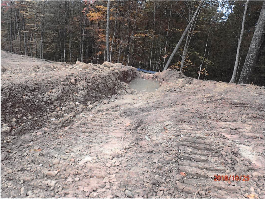
Sump at Station 286 in need of maintenance.
