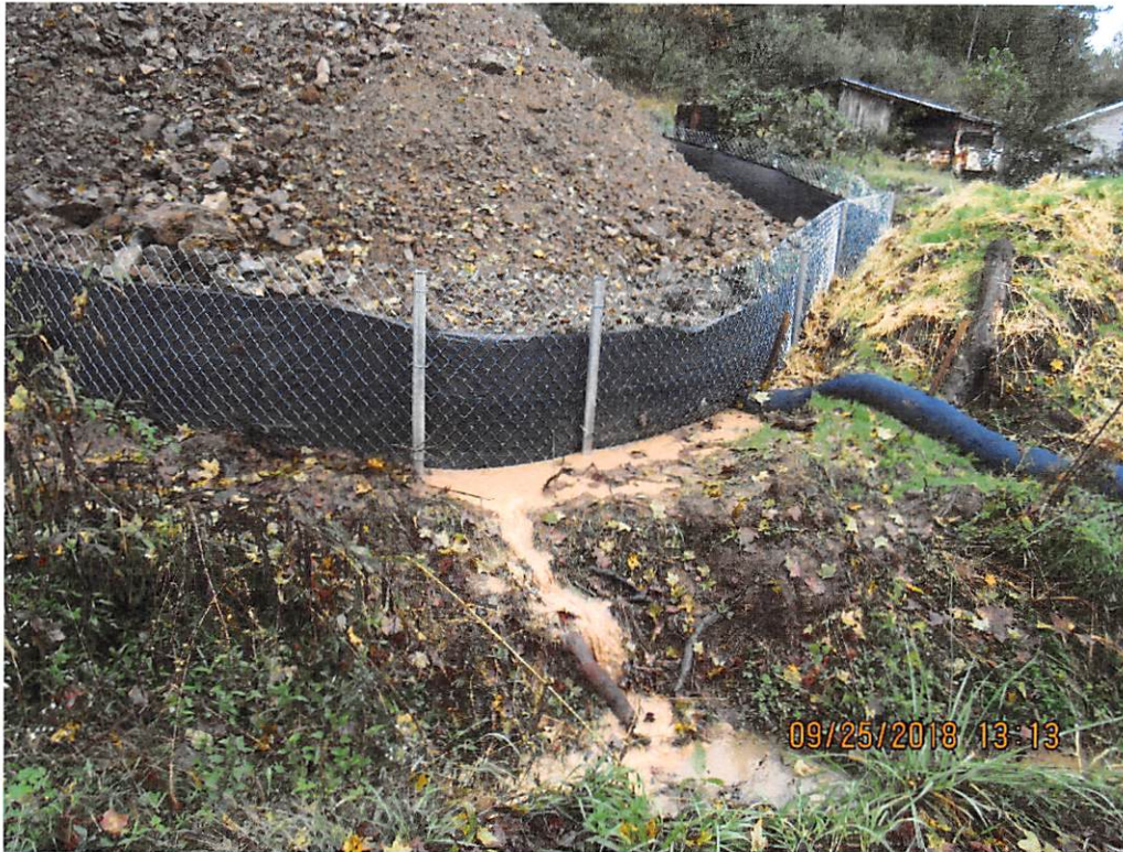
Photo 3: Failure of perimeter controls near 3634+00 allowing sediment laden water to leave site.
