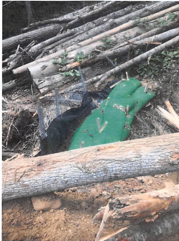
Area near station number 9907+00. Super silt fence had been undermined and damaged by logs
