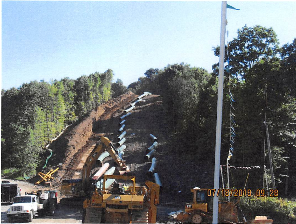
Photo 1: Station 6857+28 at access road 164 without temporary stabilization on large spoil pile. Photo is representative of project.
