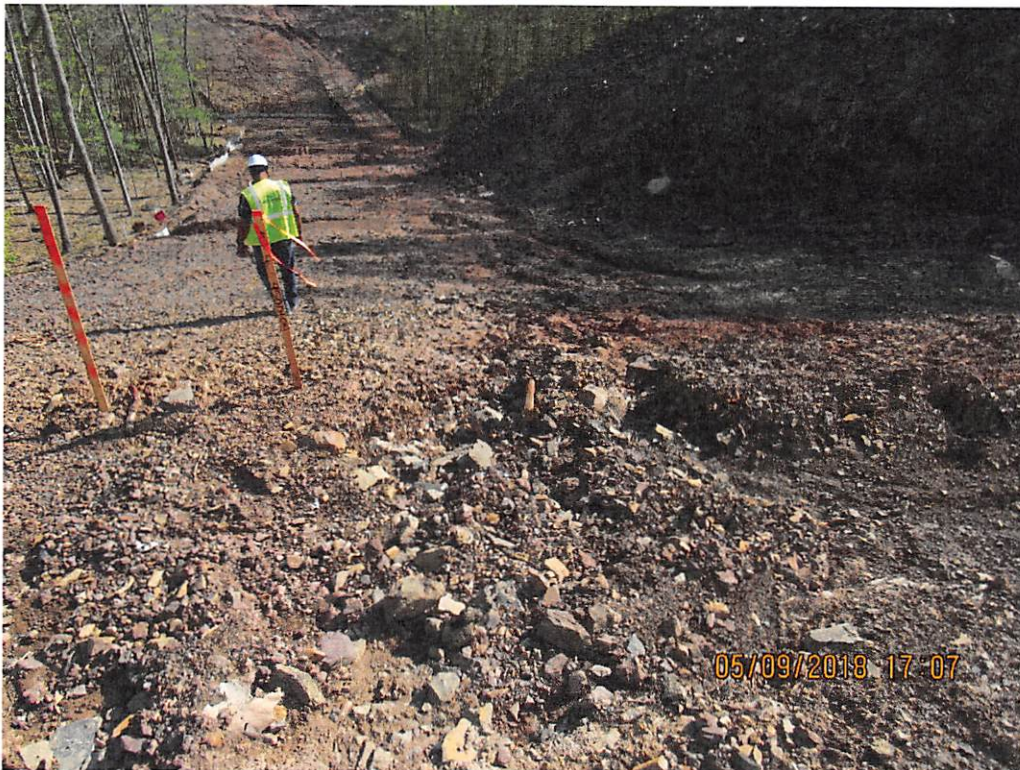
Photo 4: Downslope view of site of sediment laden water leaving site- erosion gullies observed on slope. (view south)
