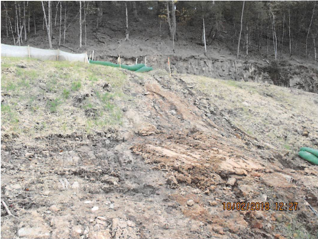
Lack of fill slope protection on opposite side of pond facing upslope near Station #9687.
