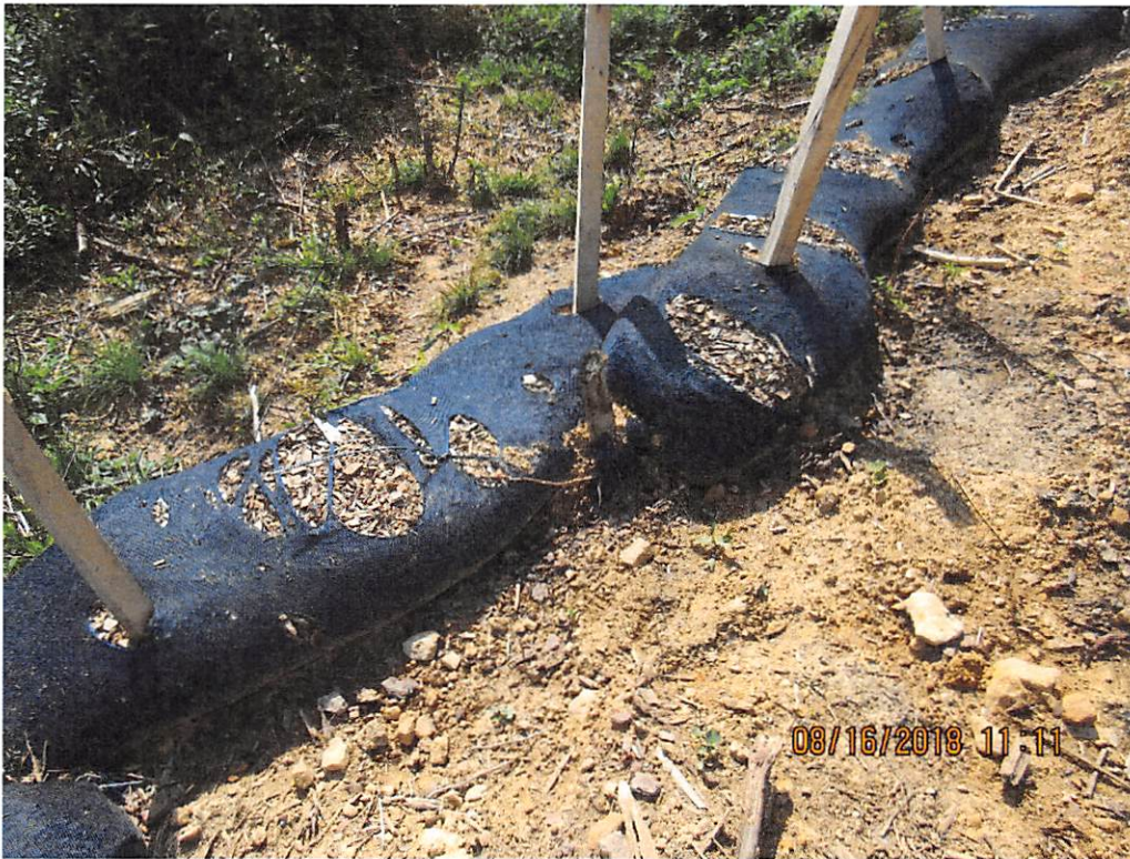
Photo 13: CFS needs maintenance near station 7232+00
