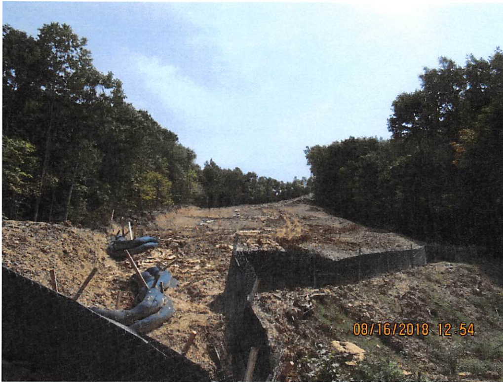
Photo 21: ROW slope between stations 7084+00- 7093+50 with inadequate number of water bars.
