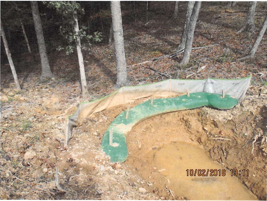
BMP outlet being overwhelmed near station number 9717+52.
