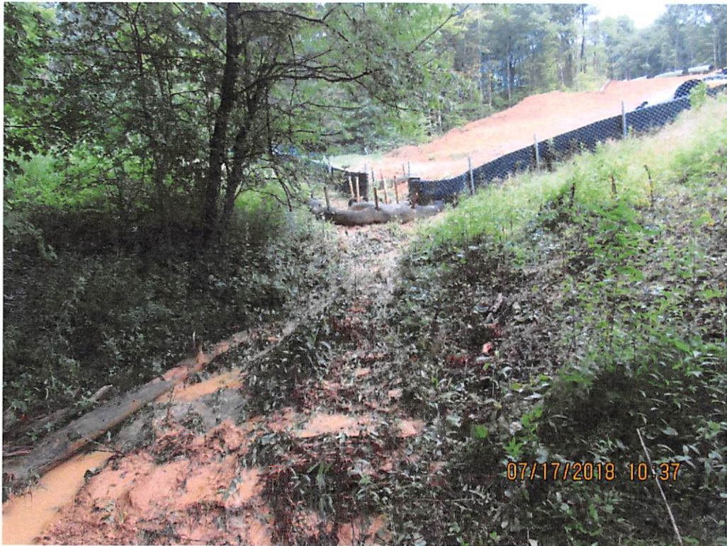
Photo 10: Upslope view of sediment deposits from control failure.
