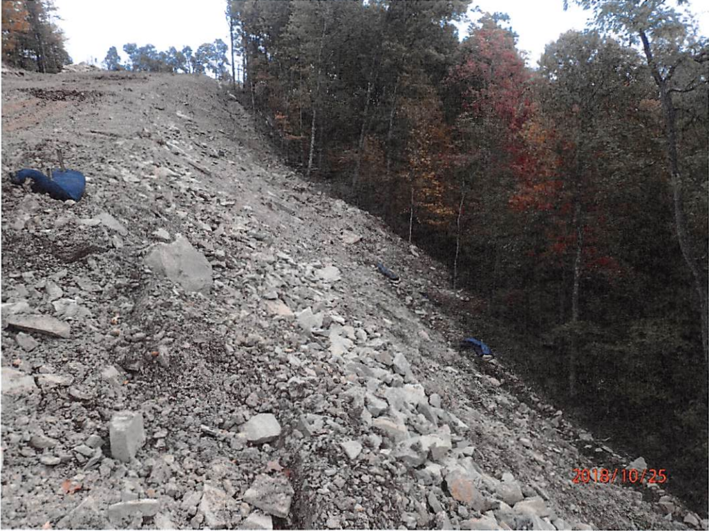
Slip at Station 489 entered the ditchline from a sideslope allowing sediment to leave the project ROW.
