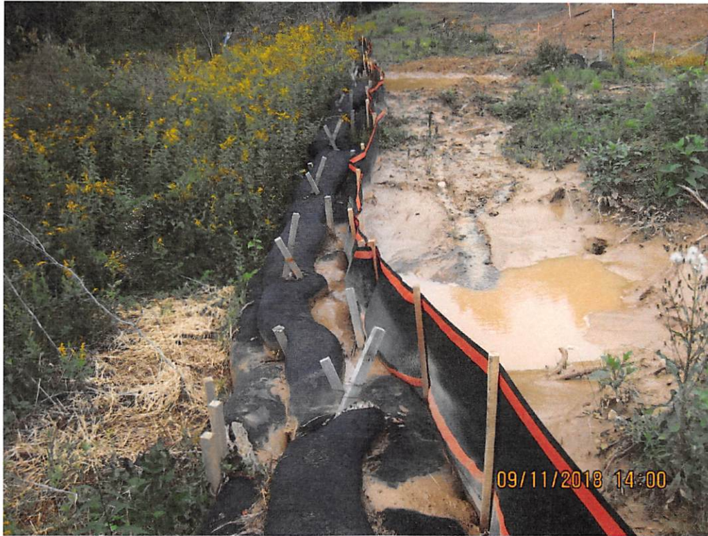
Photo 5: Station 150 (approximately)- controls maintained abating NOV issued 8/13/2018.
