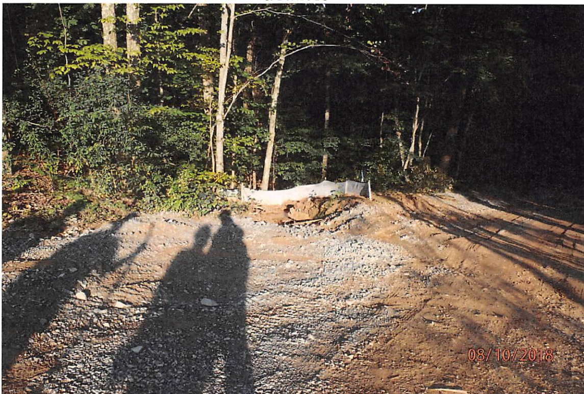
BMP that is handling stormwater from the above pictured drainage area (recently replaced).
