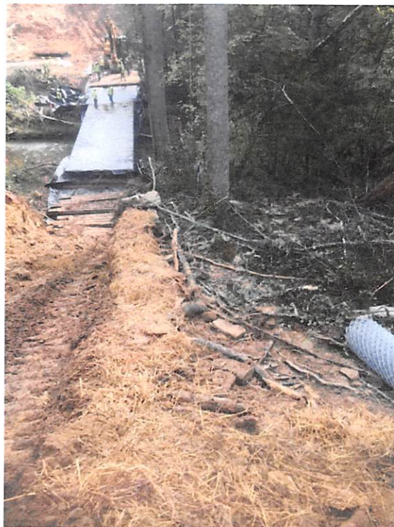
Facing Hans Creek near Station #9907+00. Super Silt fence located next to chain link had failed and sediment deposits were observed migrating towards Hans Creek.
