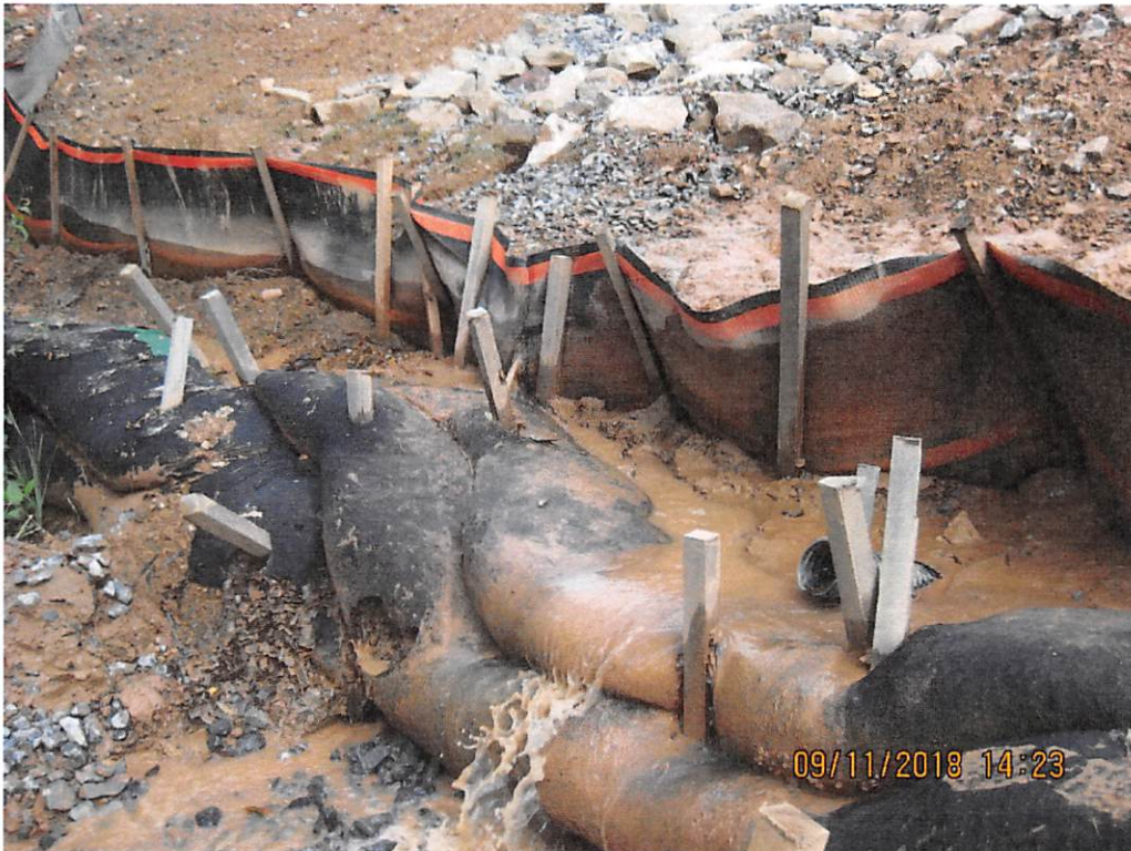
Photo 8: Station 900 (approximately)-Flow below silt fence into sump.
