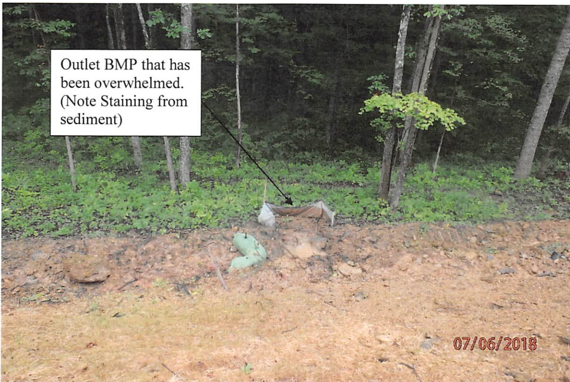
Installed temporary tight of way diversion and outlet that does not have adequate outlets adjacent to 1876+00. Evidence of the terminus BMP being overwhelmed in lower picture.
