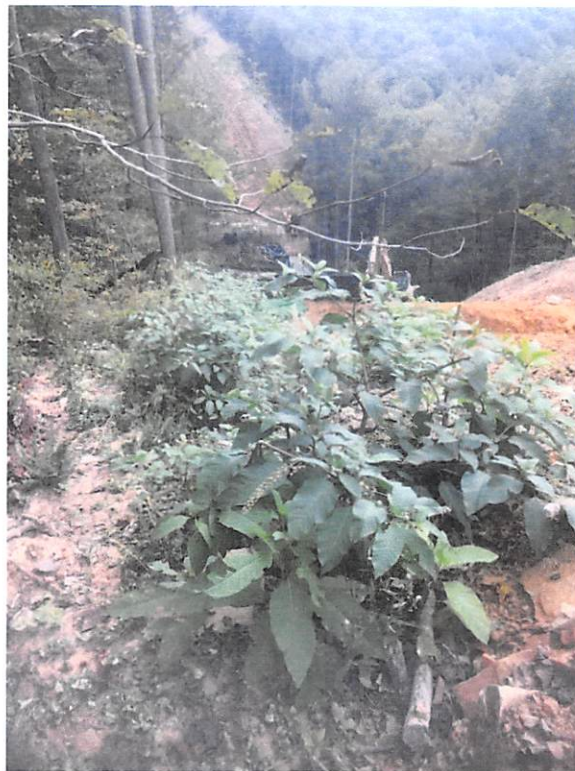
Near Station # 9911+00 where BMP was being overwhelmed and off-site sediment deposits were observed.
