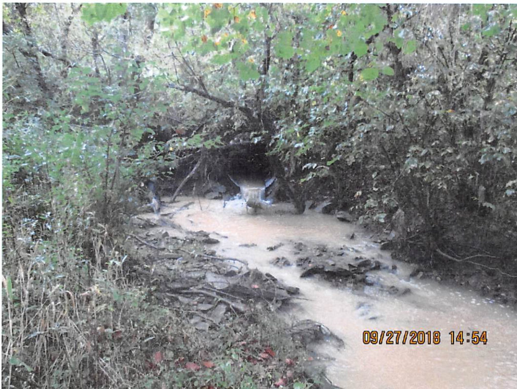
Location where sediment laden water was entering stream S-A60.
