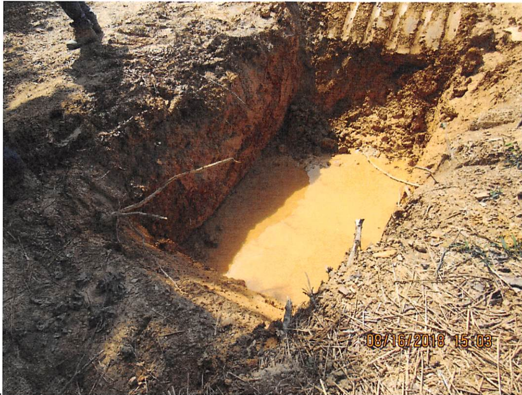
Photo 33: Recommended installation of safety fence around sumps near Wahoo Road station 6781+51.
