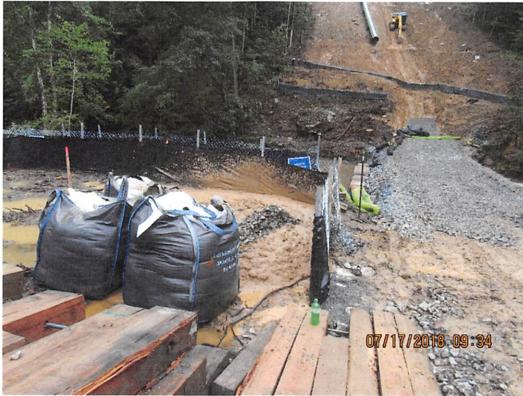
Photo 1: Sump at access road 129 needs maintenance.
