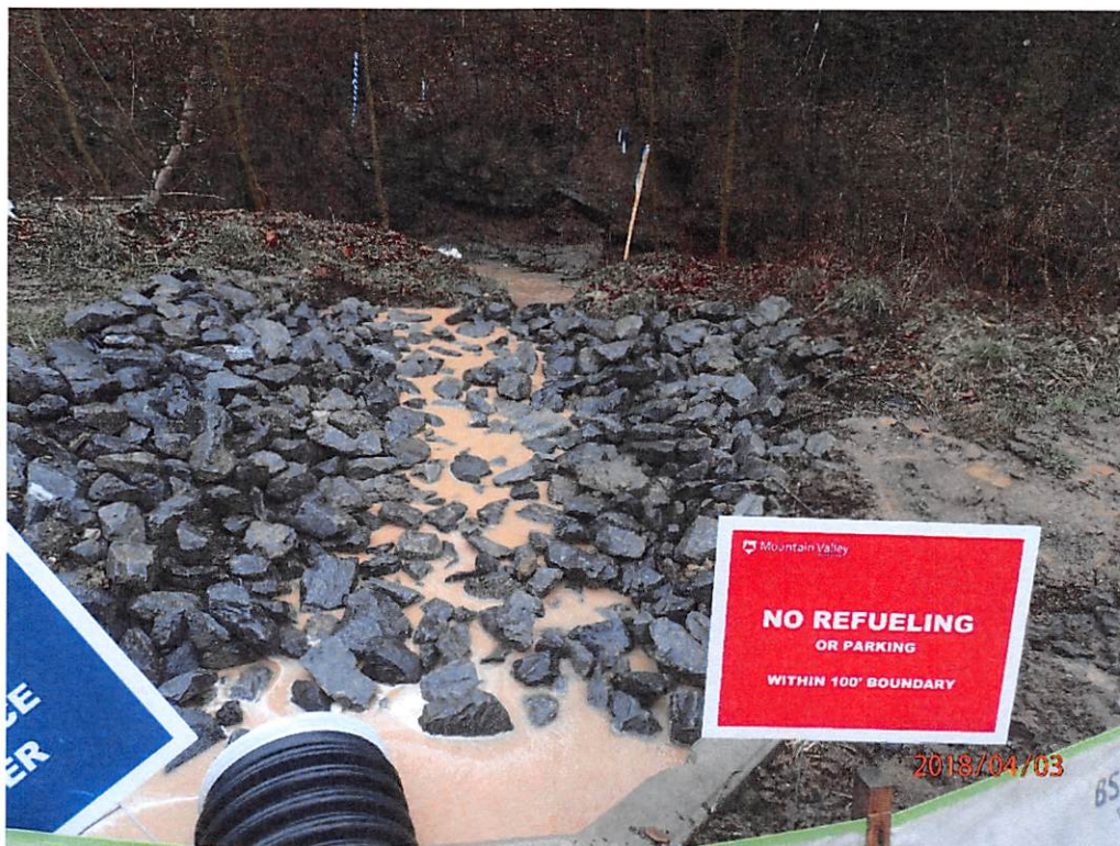
Sediment laden water leaving site into UT of Mobley Run.
