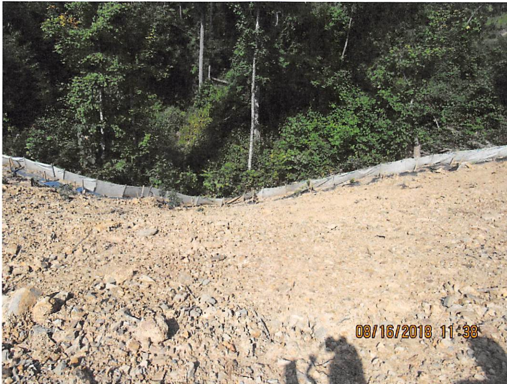
Photo 17: Inadequate controls for concentrated flow at base of fill slope near station 7158+00.
