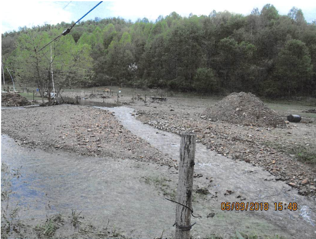
Photo 3: station 10146+32, sheet 9.35 - stream has been partially returned to channel. Rock/soil pile resulted from landowner removing debris to restore to channel.
