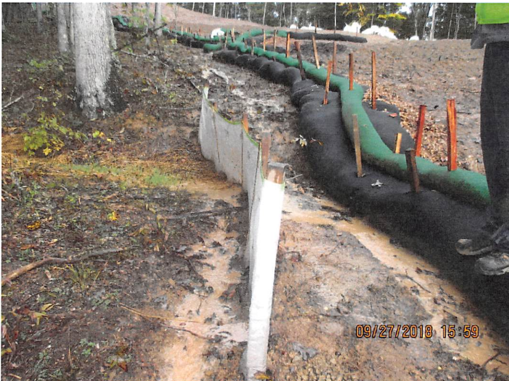
Areas near station number 9417+75 where water bar terminus being overwhelmed with sediment laden water.
