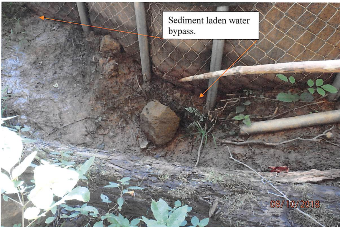
Improperly operated and maintained BMP at a water bar terminus in the Meathouse Fork watershed that led to CNA deposits and distinctly visible settleable solids in UNT Meathouse Fork (39° 11.891' X 80° 33.209').
