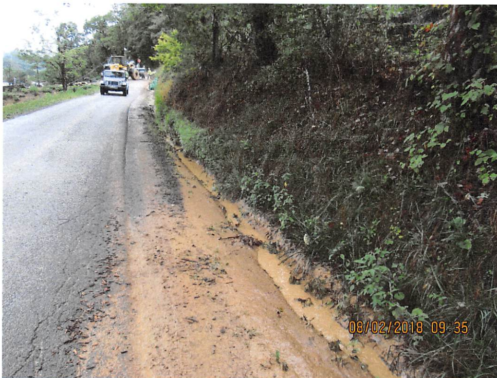
End of road side ditch prior to culvert diverting to laydown yard.
