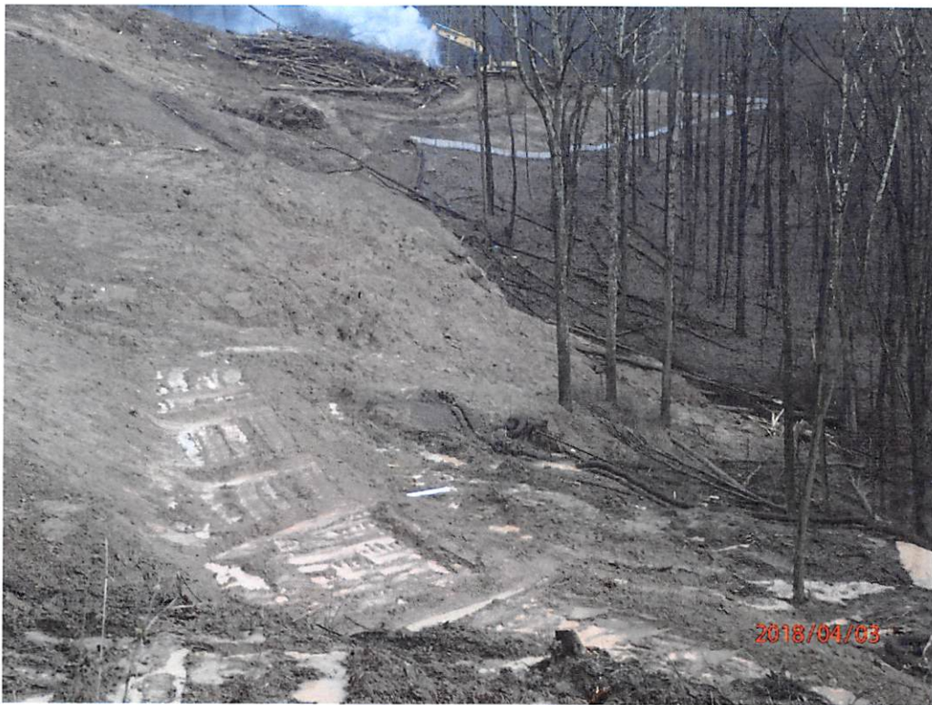
Reported slip area near Bradshaw Compressor Station.
