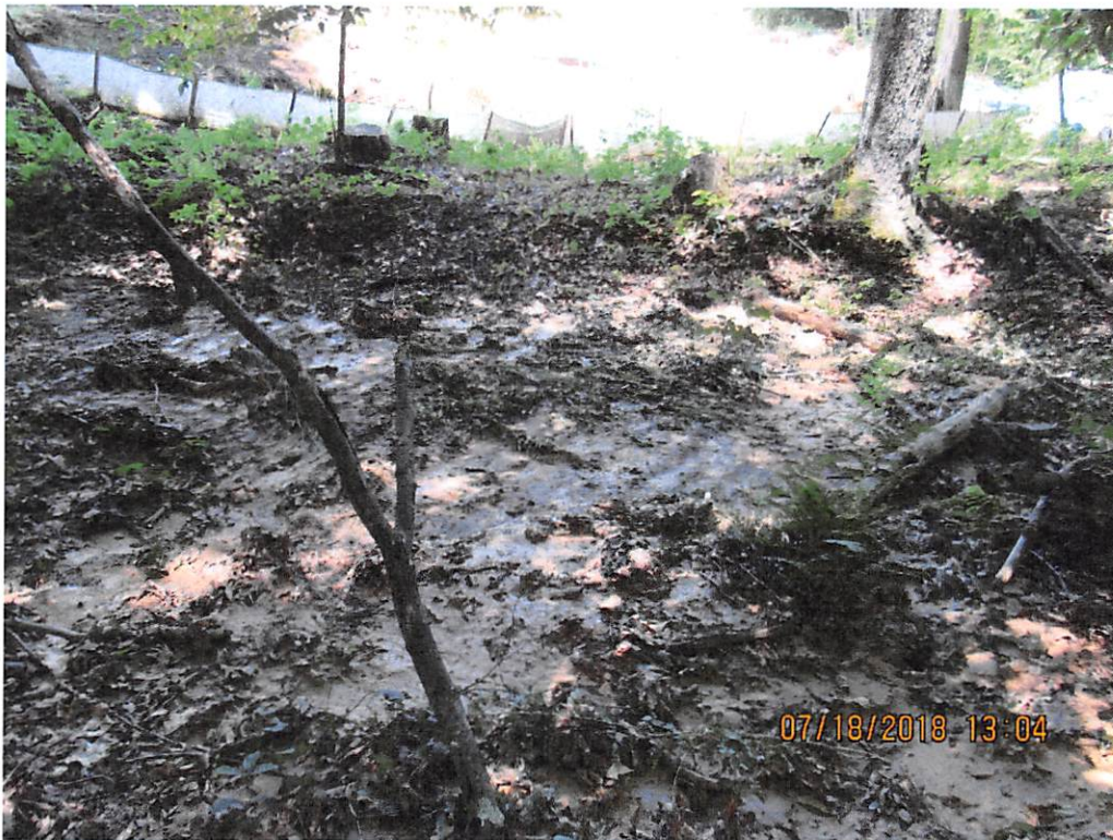
Photo 14: Sediment deposits off limits of disturbance from station 6785+50 control failure.
