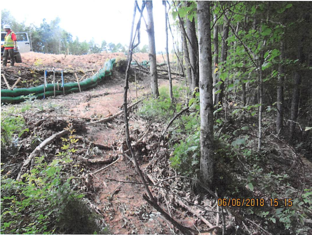
Photo 6: Continued scoured path from control failure at station 6812+58.
