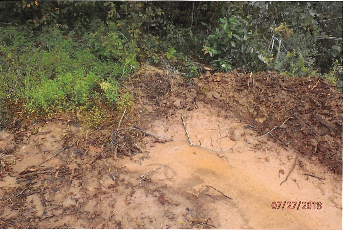
Water bar that lacked outlet protection was noted upslope of grass run adjacent to 1142+00.
