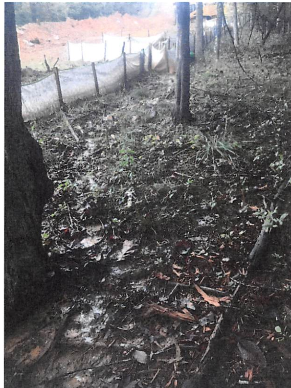
ROW near station numbers 9779+00 and 9778+00 where water bar outlets were being overwhelmed and sediment laden water was passing through and under and being transported past LOD.
