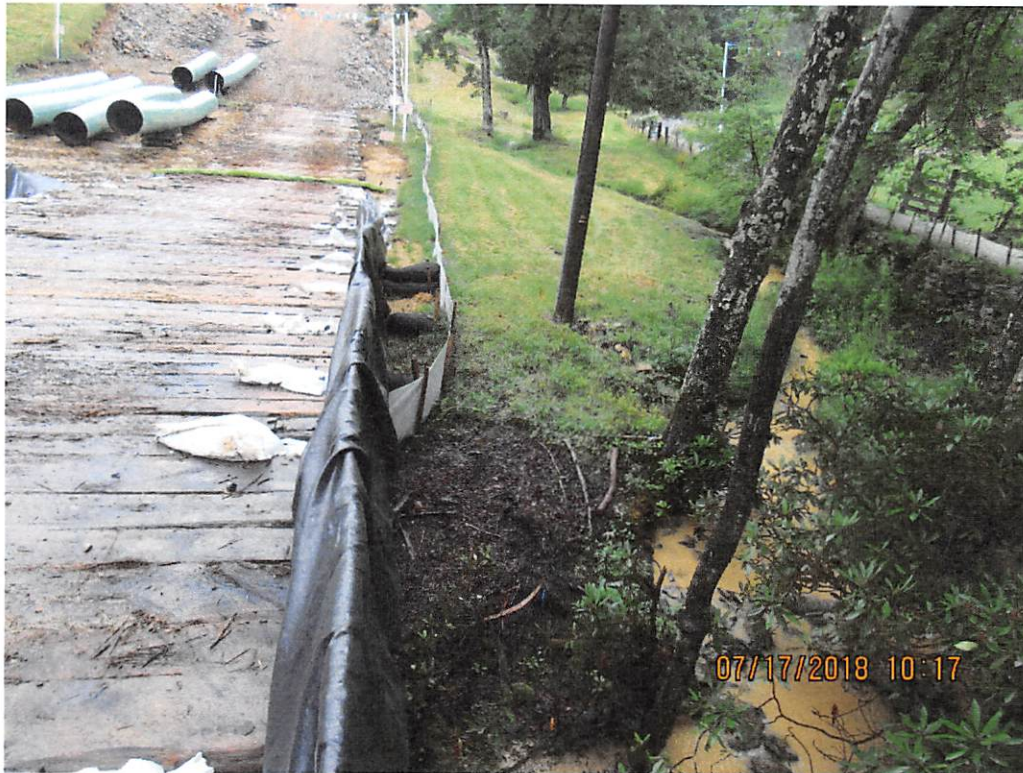
Photo 11: UNT #2 of Birch River (S-F365) at station 5548+00 where breached control upstream allowed sediment laden water in UNT #1 of Birch River (S-F34)
