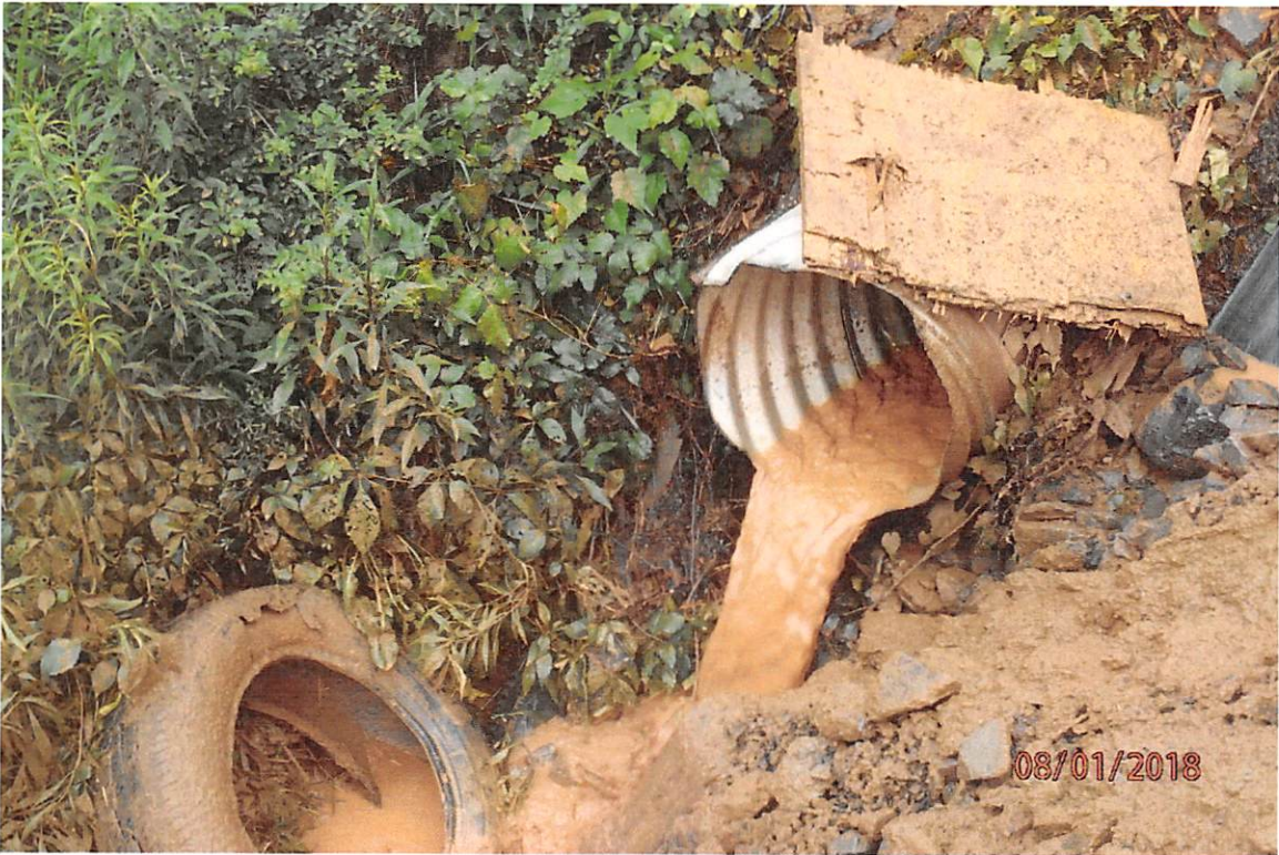
Sediment laden water that is bypassing the installed BMPs due to improper BMP operation and installation.
