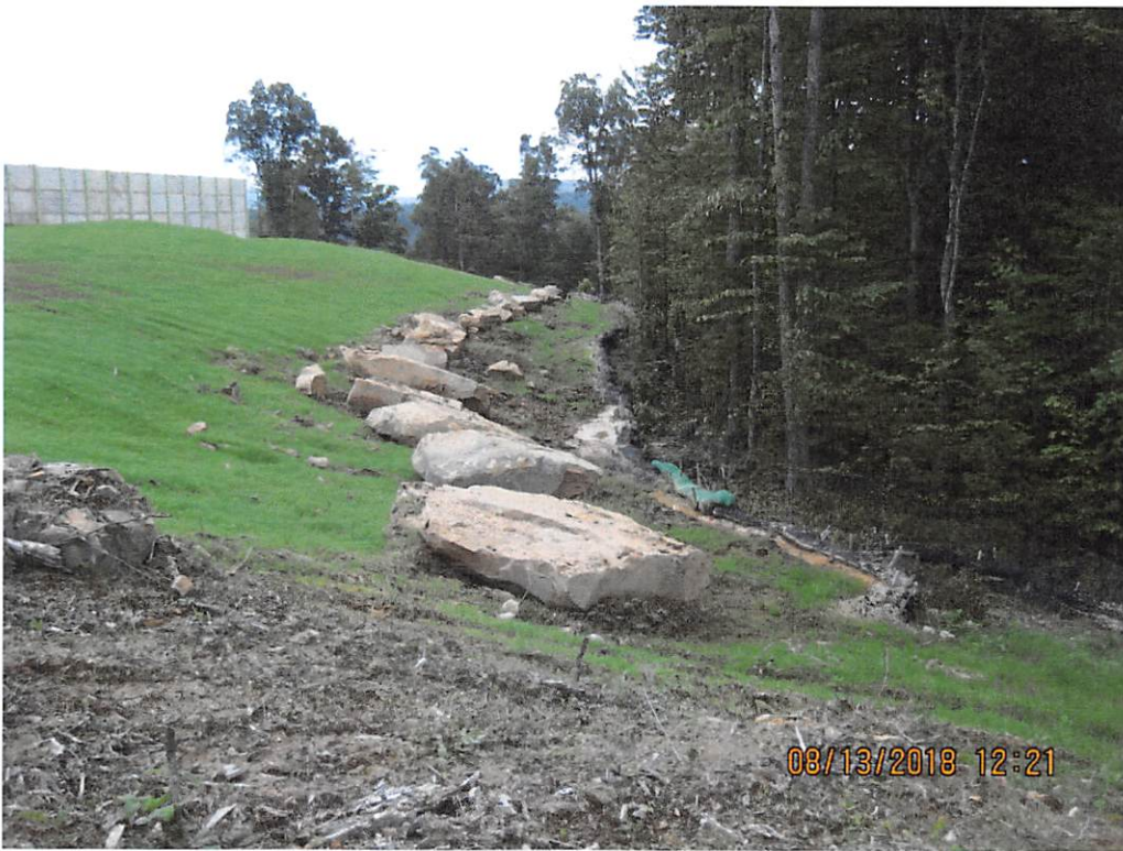
Maintenance needed for filter sock at Southwest wall.
