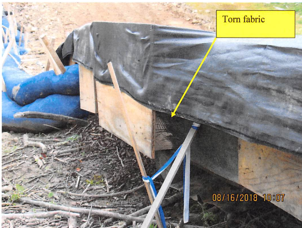
Photo 10: Exterior view of punctured fabric in Photo 9.
