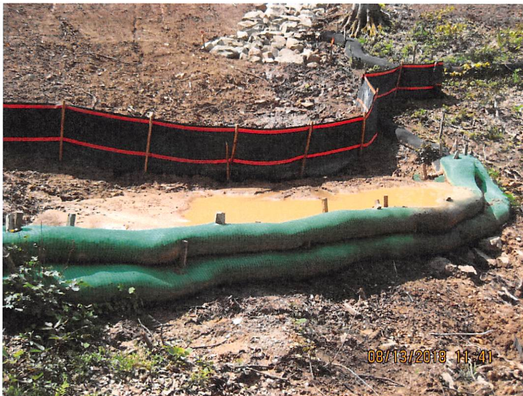
Maintenance needed north of the east wall.
