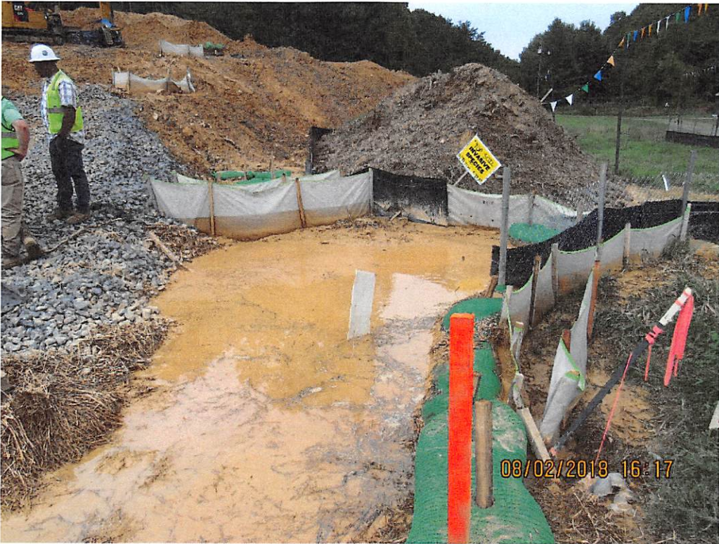
Station 10270+00, sump is full.
