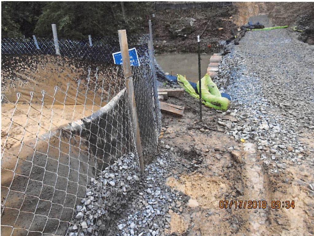
Photo 2: Proximity of outlet of sump and amount of accumulated sediment creates an area of concern.
