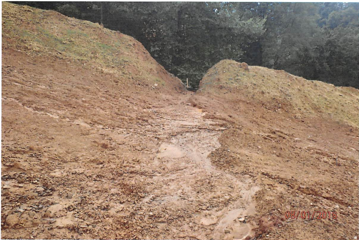
Improperly installed and poorly maintained water bars in the Goose Run watershed.
