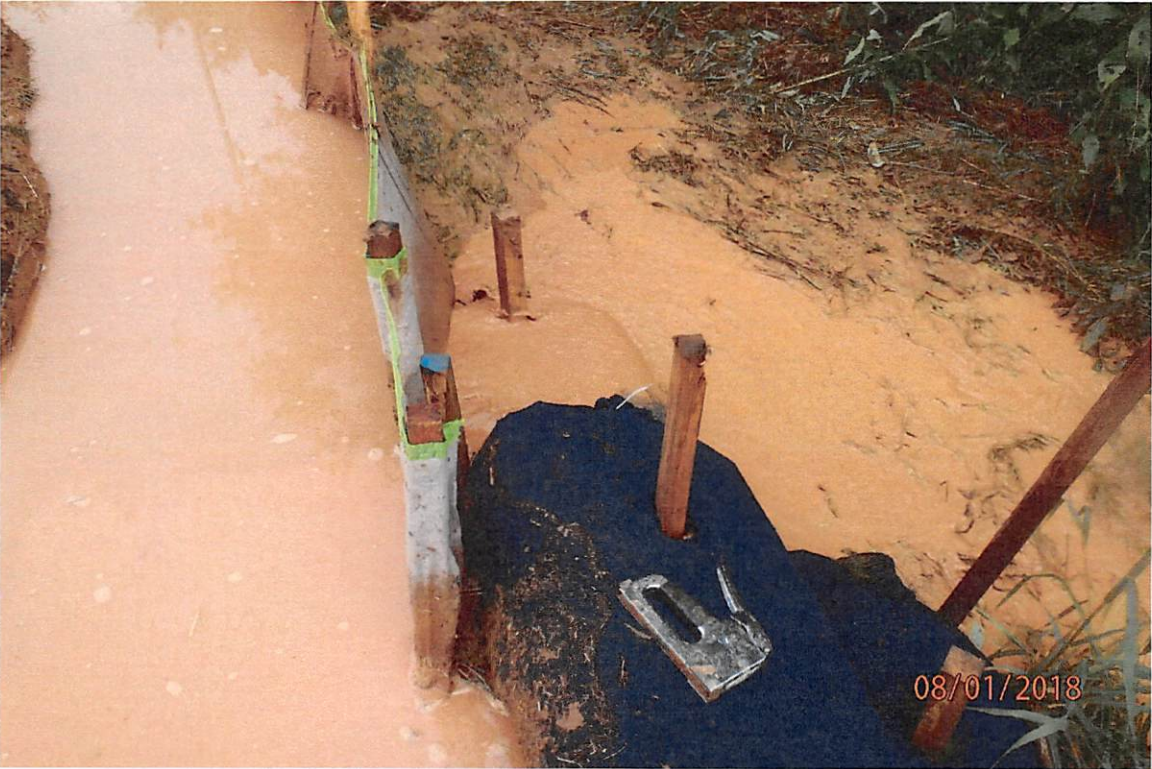
Improperly operated BMP that is causing sediment laden water to leave the site and CNA visible in Big Elk Creek.
