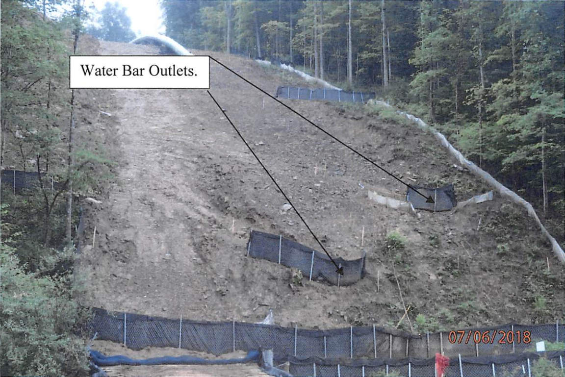
Water bars that are not installed properly and do not shed stormwater off of the LOD in small quantities as designed located adjacent to Laurel Run of Meathouse Fork crossing.
