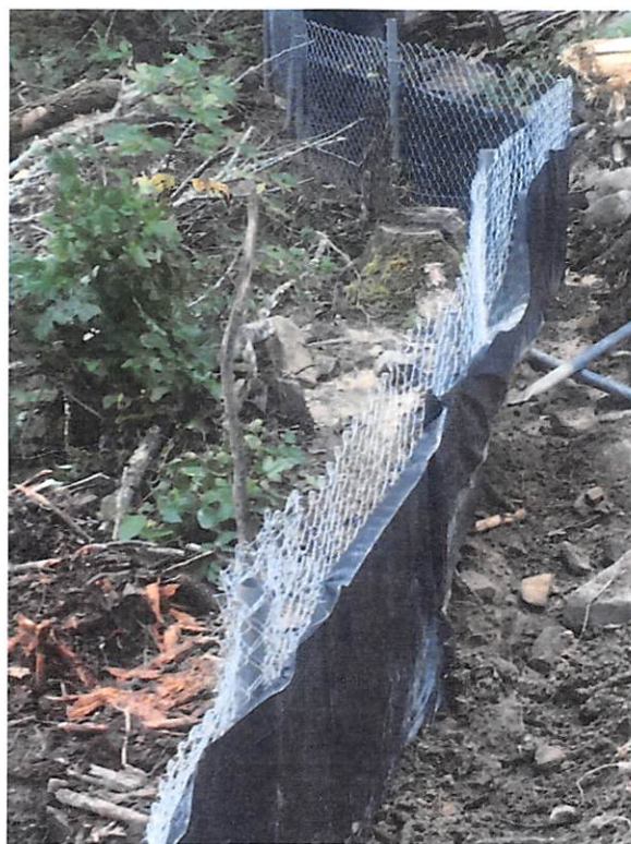
Area near station number 9907+00. Super silt fence had been undermined and damaged by logs.
