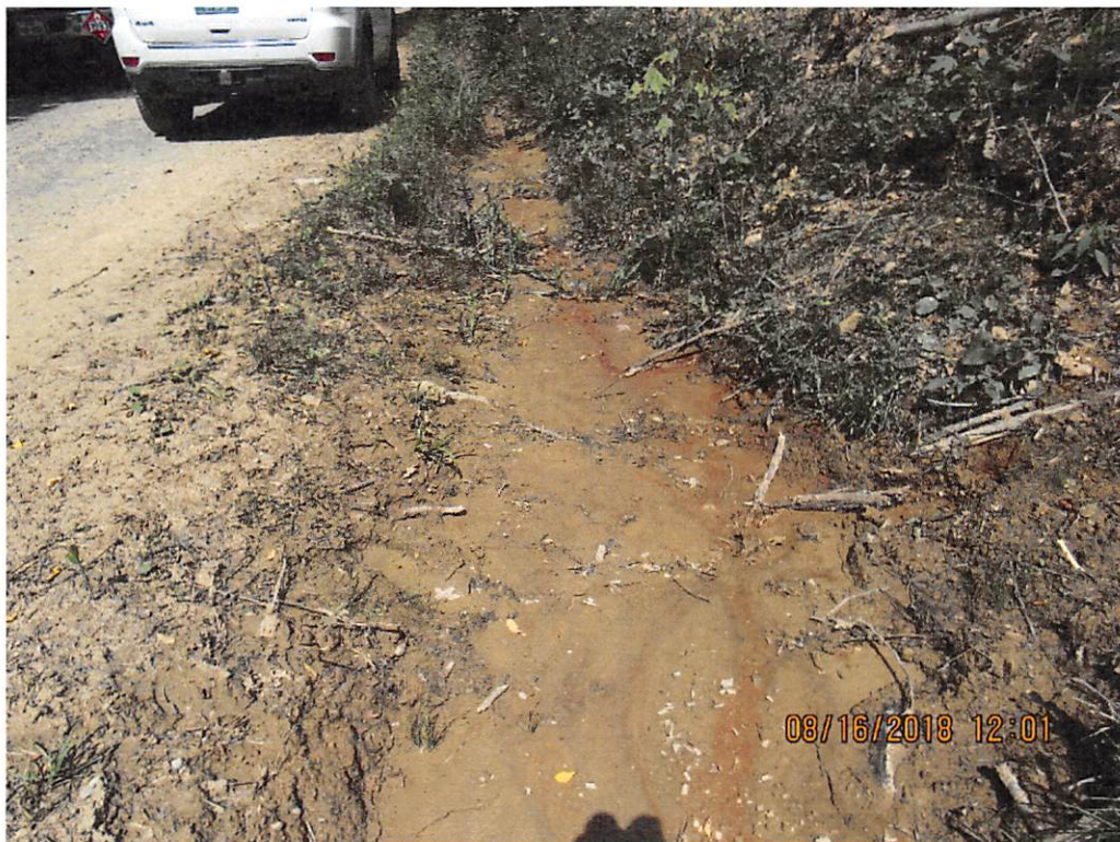
Photo 26: Road side ditch below water bar terminus in photos 23-25 conveying sediment laden water to installed culvert.
