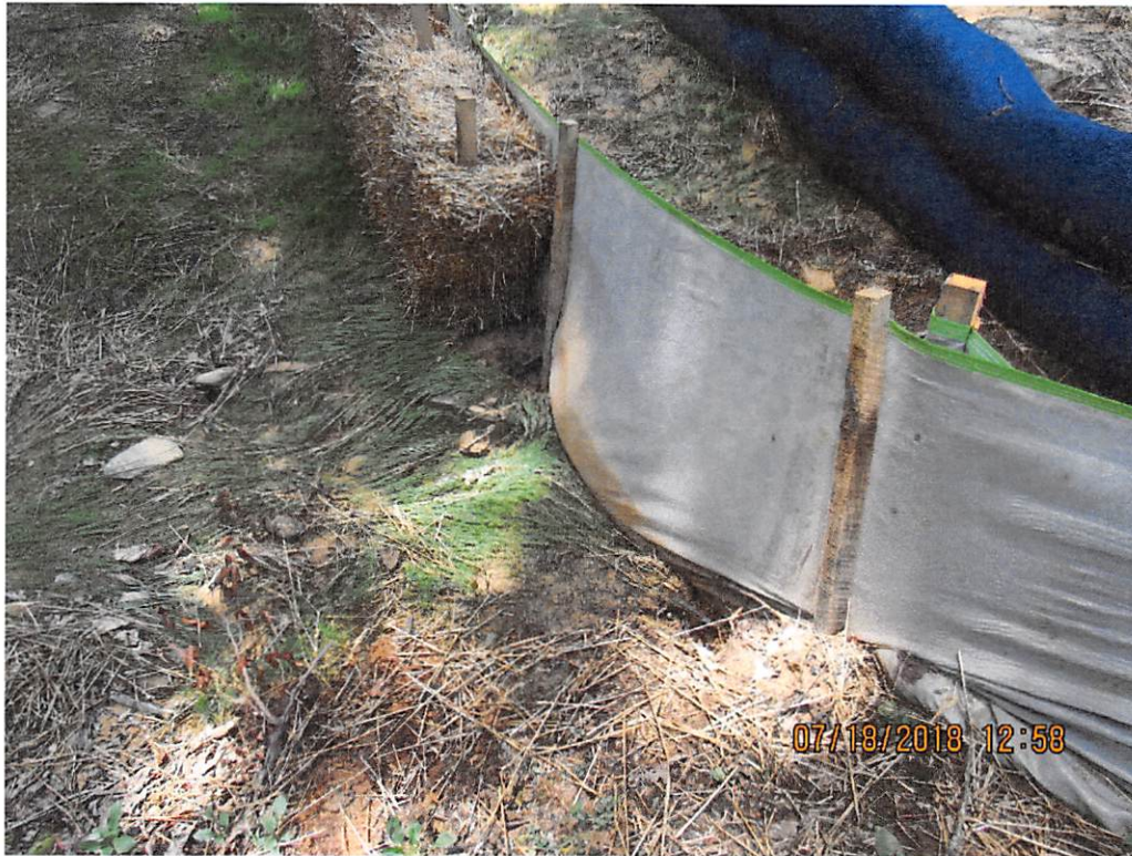
Photo 11: Down gradient of control failure from Photo 10. Photo #7 shows terminus of this control failure.
