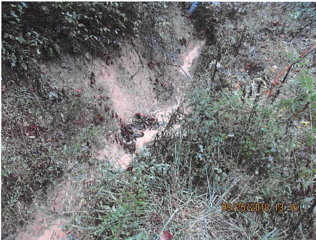
Photo 1: Sediment laden water from sumps near station 3625+00.
