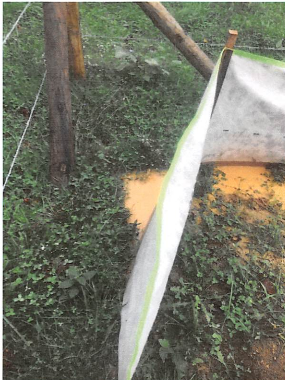
Sediment laden water flowing under and through BMP near station number 9784+00.
