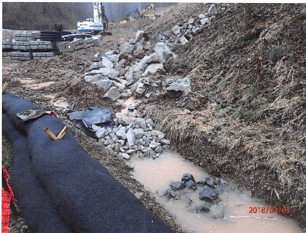
Sediment laden water leaving site through drop inlet.
