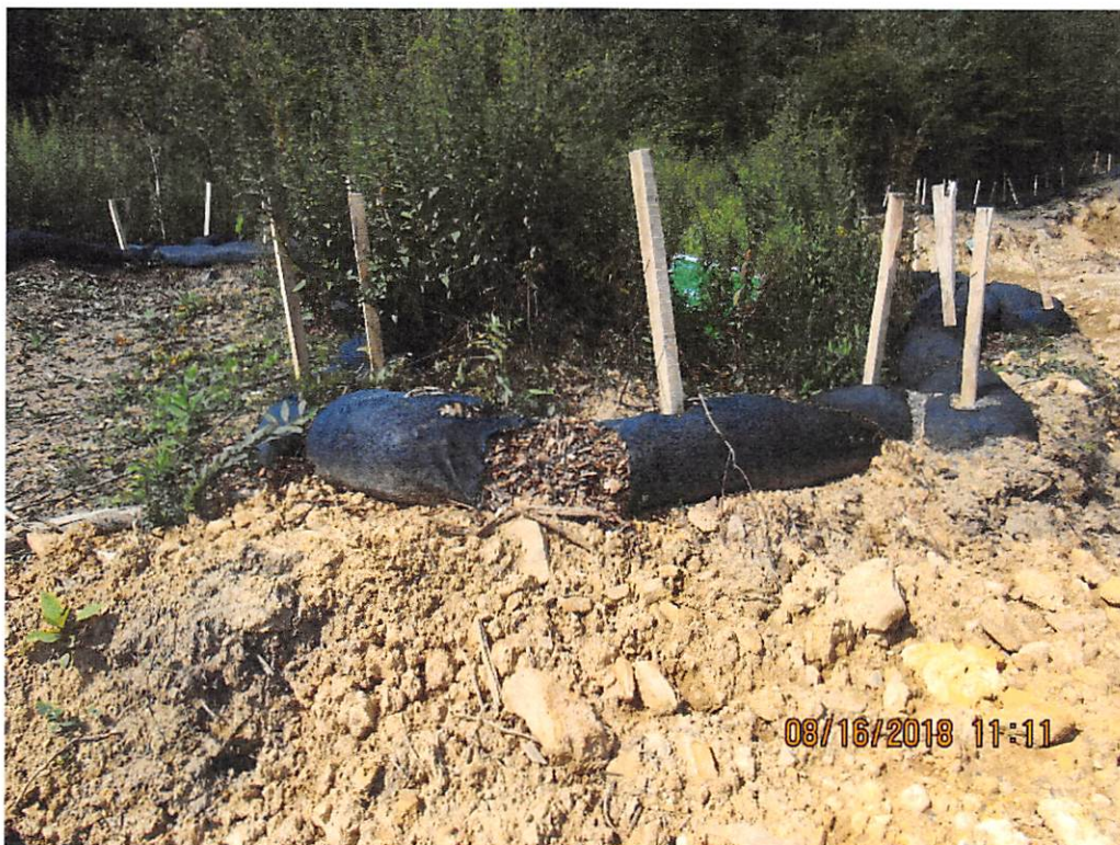
Photo 14: CFS needs maintenance near station 73232+00.
