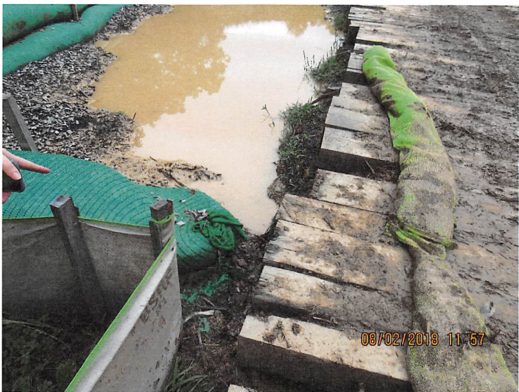
Source of sediment laden water in Slate Run.
