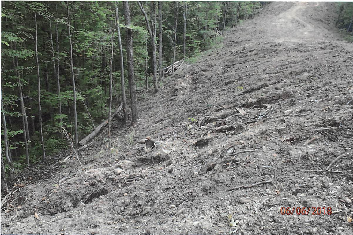
Areas of the project that have been cleared to mineral soil and BMPs are not in place as indicated in the SWPPP.
