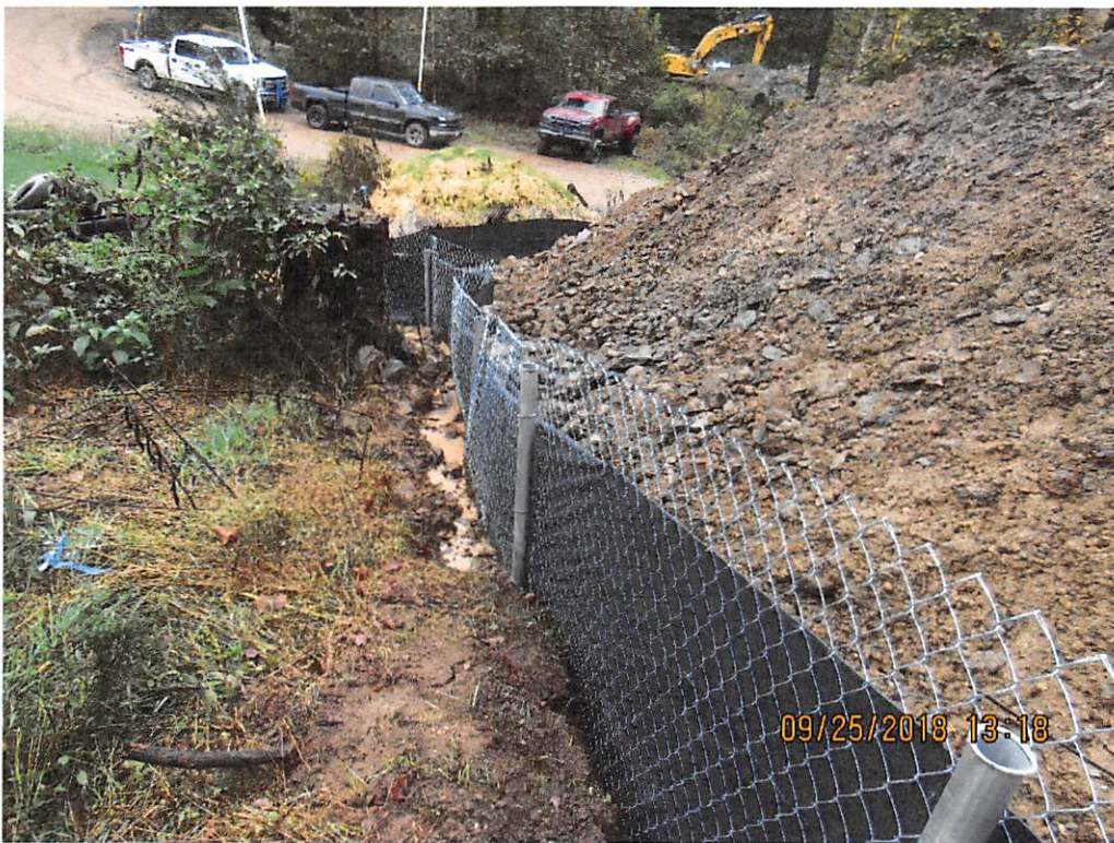
Photo 2: Undermined perimeter controls near 3634+00 which failed allowing sediment laden water to leave site.
