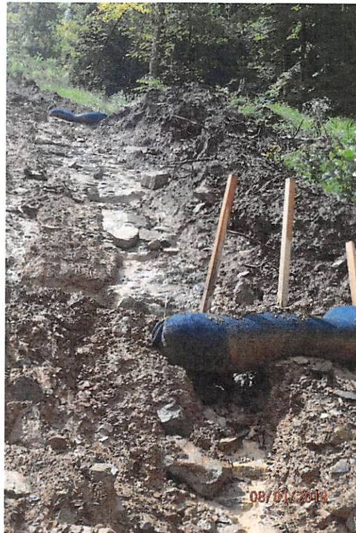
Improperly installed water bars that have caused fill slope erosion in the Big Elk Creek watershed.
