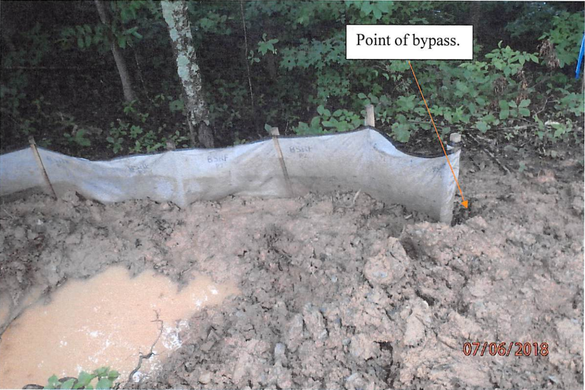
Improperly installed BMP at the terminus of a water bar adjacent to MVPDO-049 (1891+00) that allowed sediment laden water to leave the site and caused CNA in UNT Dry Fork.
