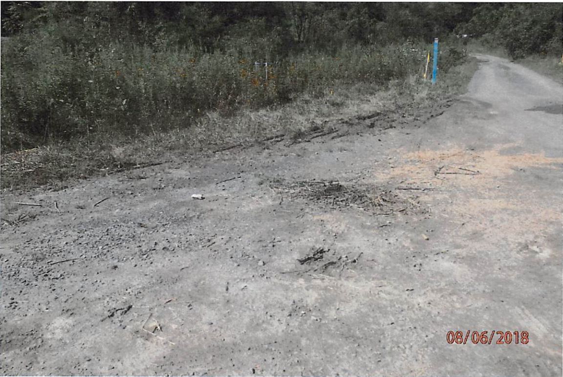
Area adjacent to wetland (W-UU1) in the Salem Fork watershed that lacks the BMPs that are indicated in the approved SWPPP.
