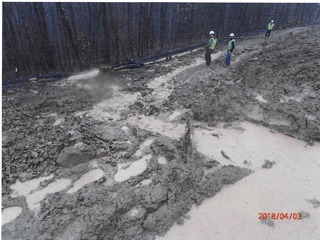
Third site of sediment laden water leaving site at Bradshaw Compressor Station.
