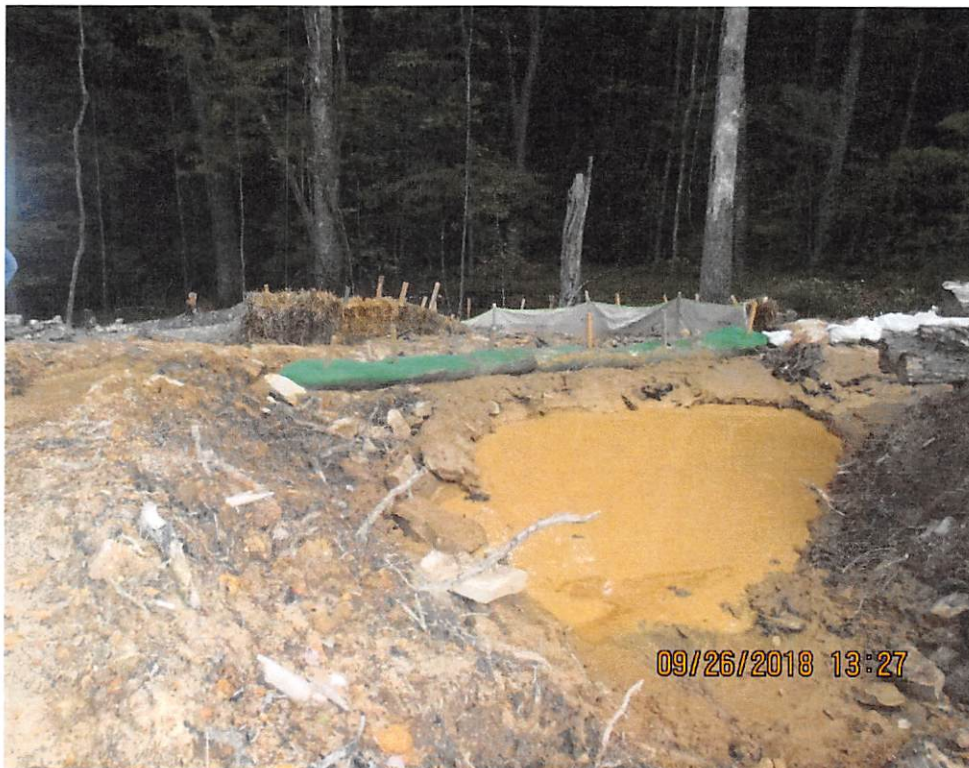
Waterbar terminus near being overwhelmed near Station #9899+00.
