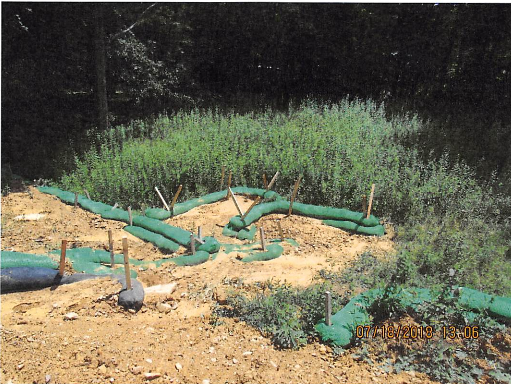
Photo 18: Installed controls at end of water bar proved inadequate and failed allowing sediment laden water to leave site.
