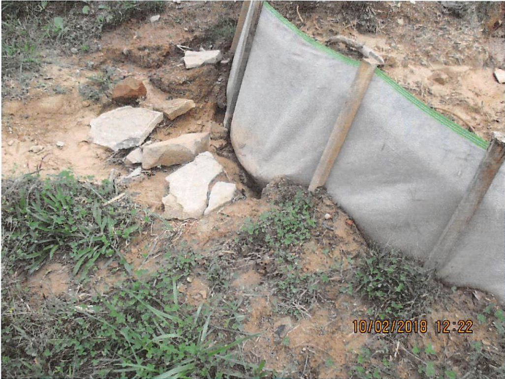
Above mentioned BMP being undercut from run-off.
