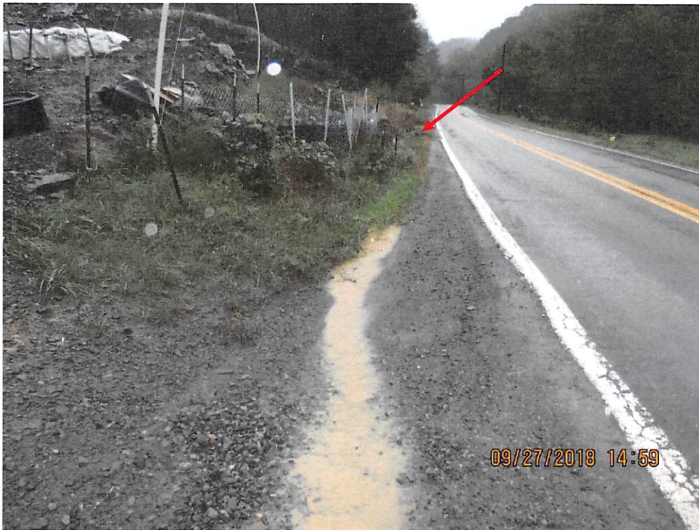
Sediment laden water leaving ROW intercepted by ditch flowing towards Stream (S-A60). Arrow depicts where ditch connects to stream S-A60 and flows under road via culvert.
