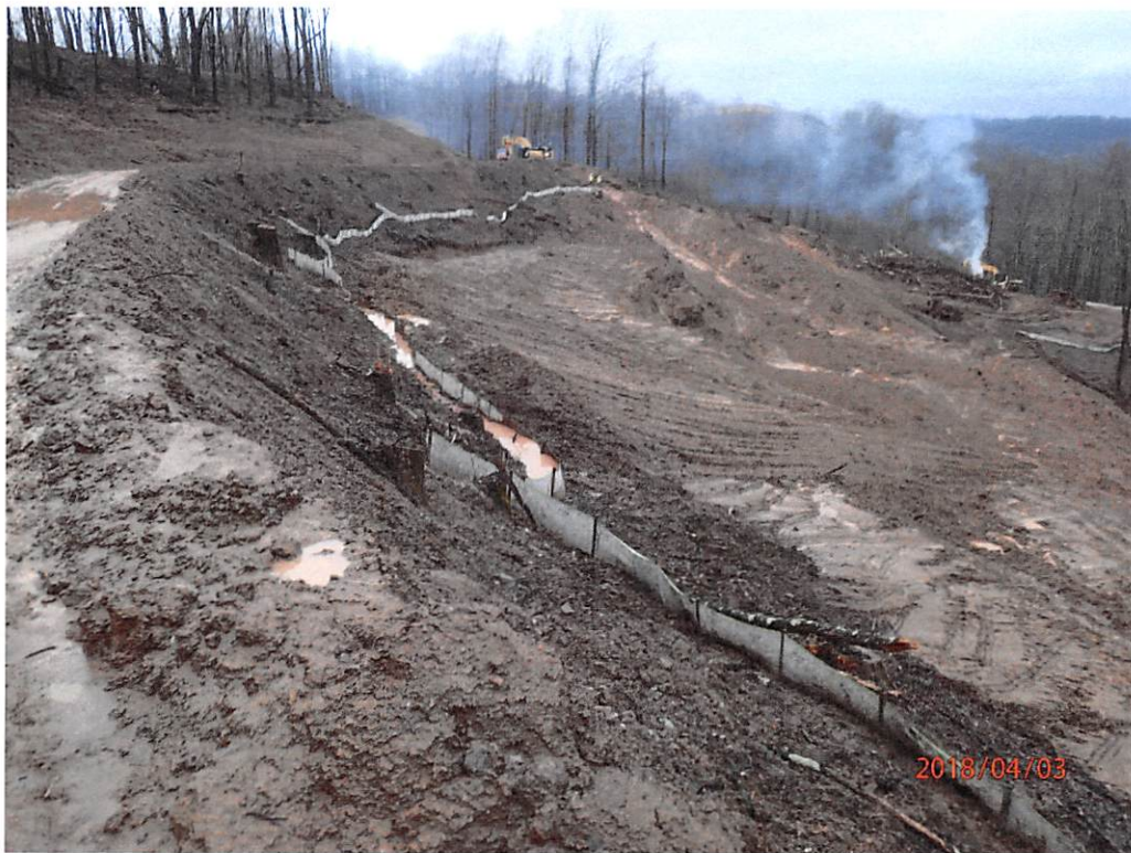
Hillside above slip near Bradshaw Compressor Station.
