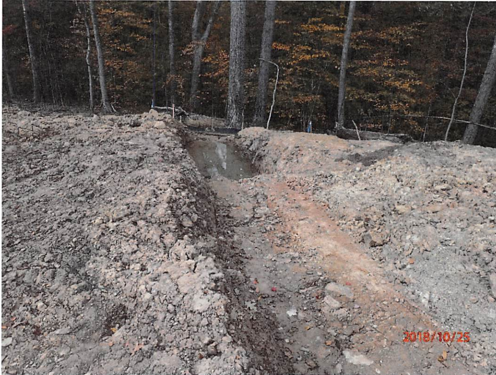
Sump at Station 290 in need of maintenance.
