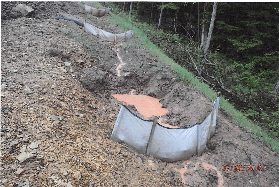
The installed temporary right of way diversion and outlet adjacent to 1851+00 that was collecting stormwater from multiple water bars without adequate outlets. This caused concentrated flow to overwhelm the installed BMP at the base of the slope.
