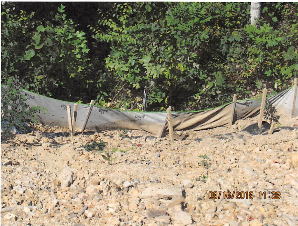
Photo 18: Close-up of inadequate controls for concentrated flow at base of fill slope near station 7158+00.
