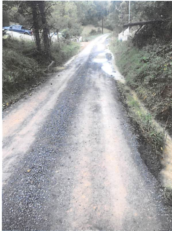
Photo looking down Ellison ridge road towards culverted stream crossings S-Z5 and S-Z4.
