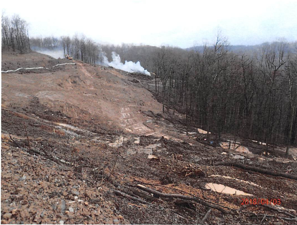
Disturbed area near the reported slip area.
