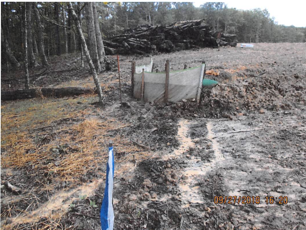
Sediment laden water flowing past BMP near Station #9417+75
