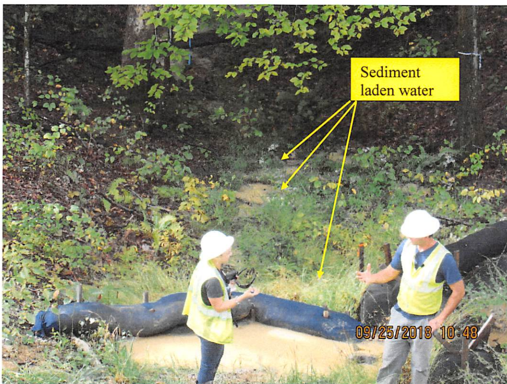
Photo 2: Station 550 sump at base of fill slope where perimeter controls failed and sediment laden water leaving site.
