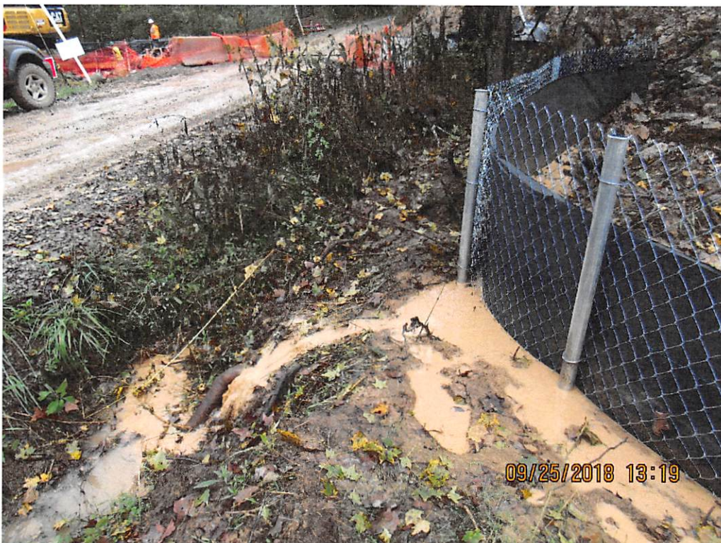
Photo 4: Close-up of failed perimeter controls near station 3634+00 where sediment laden water is entering UNT of Knawls Creek.
