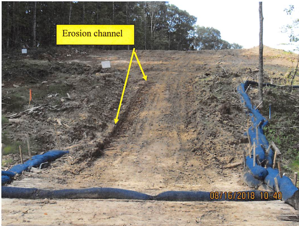
Photo11: Entrance off Bingham Road (station 7450+00) with inadequate slope breakers near stream.
