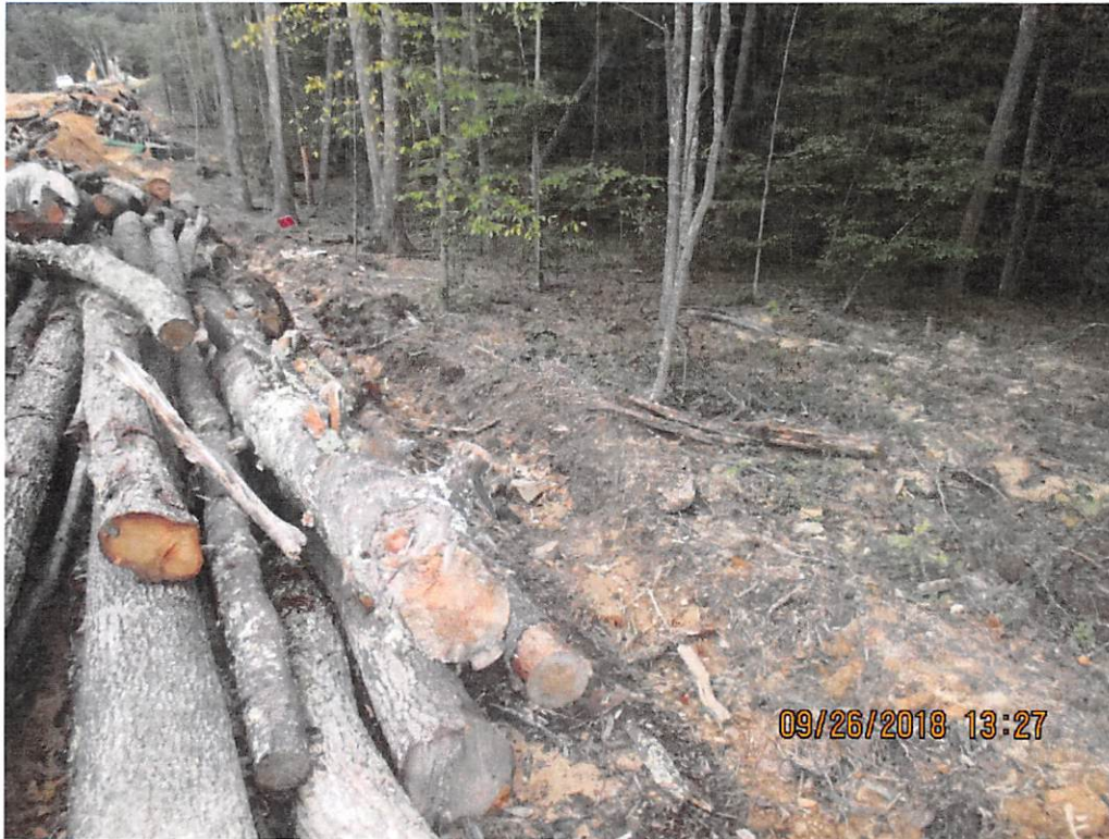
Off-site sediment deposits near Station number 9899+00.
