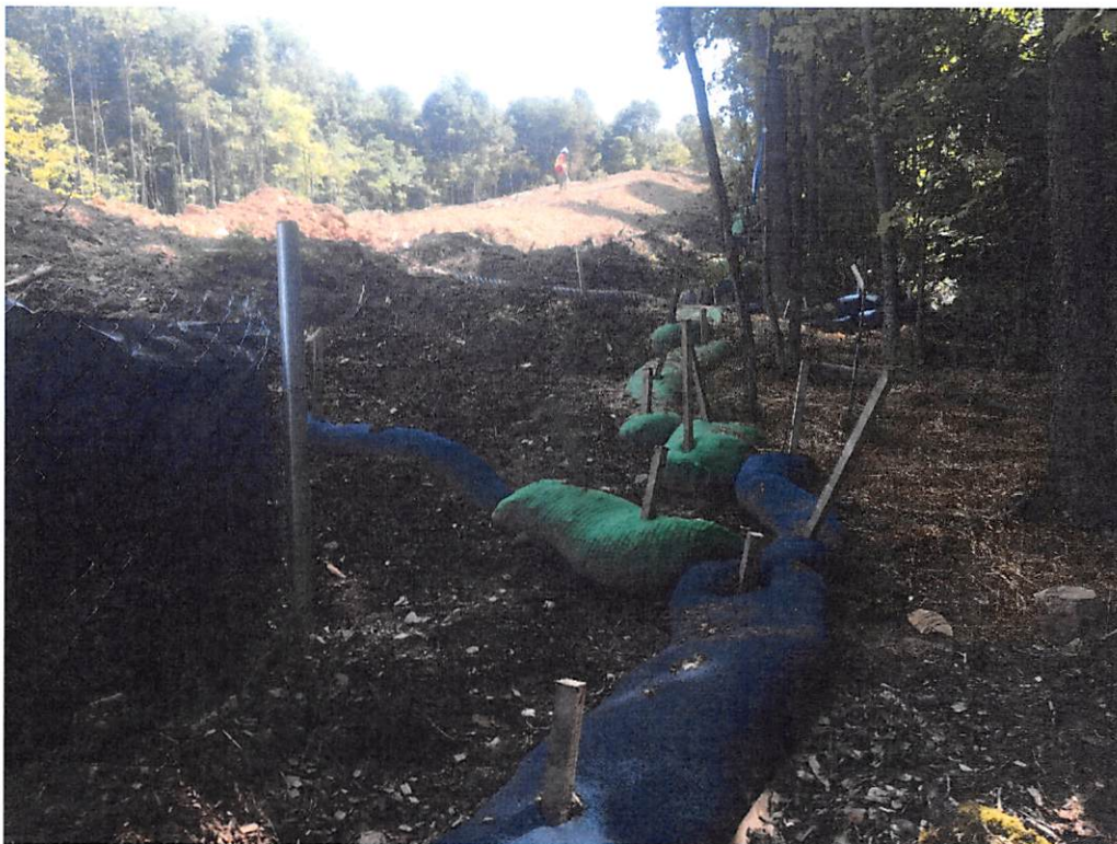
Photo 22: Failure of installed water bars between stations 7084+00 – 7093+50.
