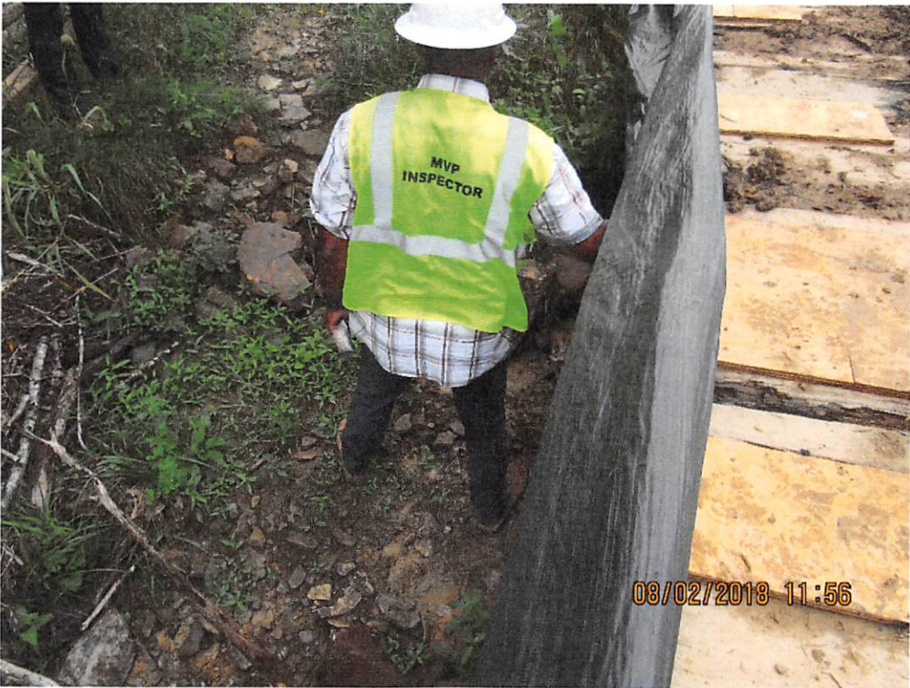
Sediment deposits observed below base of Slate Run bridge.
