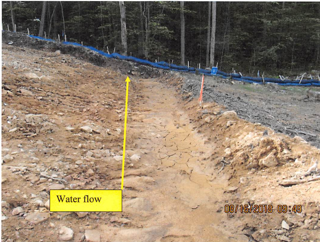
Photo 3: Incorrectly sloped water bar at Bingham Road station 7450+00- water is flowing away from outlet.
