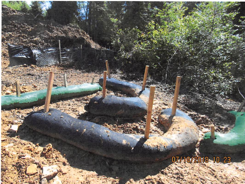
Photo 2: Controls at end of water bar were over topped at station 6898+59.
