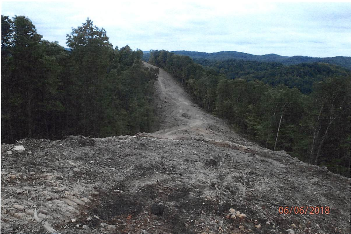
Areas of the project that have been cleared to mineral soil and BMPs are not in place as indicated in the SWPPP.
