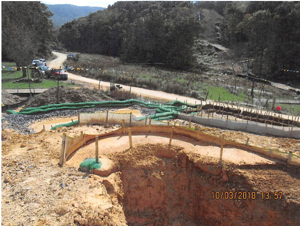
Photo 3: Front of control on right in Photo 2 after maintenance performed at Painter's Run station 10270.
