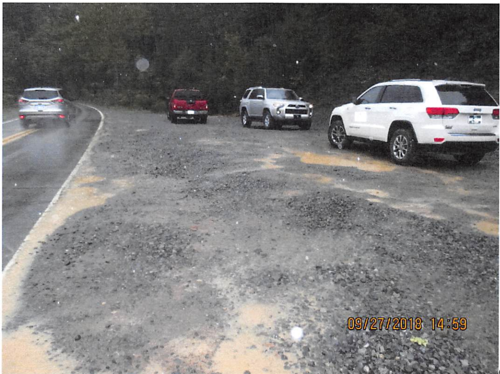
Sediment laden water accumulating and draining towards roadside ditch that intersects with S-A60 along Route 122.
