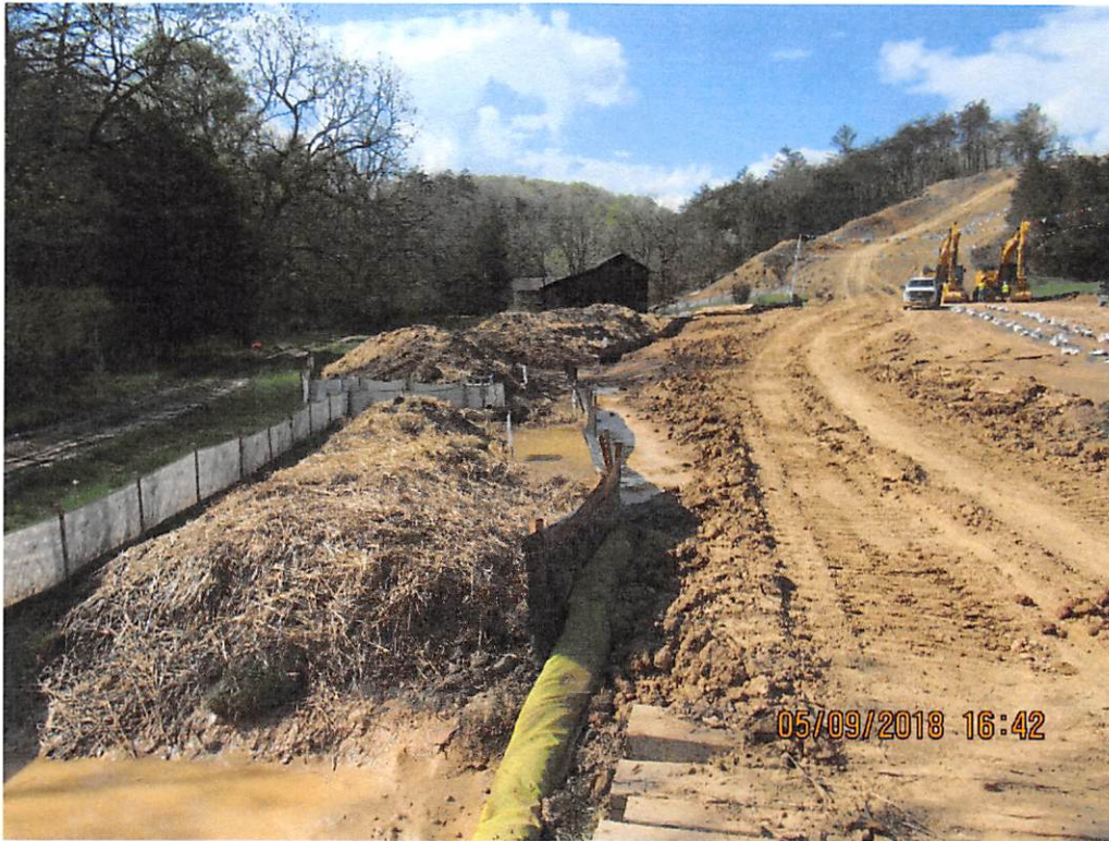
Photo 1: Delineation of topsoil stockpiles from subsoil with black silt fence and path to sump prior to stream.
