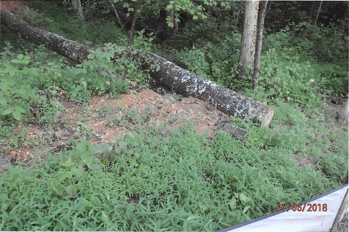
Water bar that has been installed at a steep angle with erosion and the associated offsite sediment deposits.
