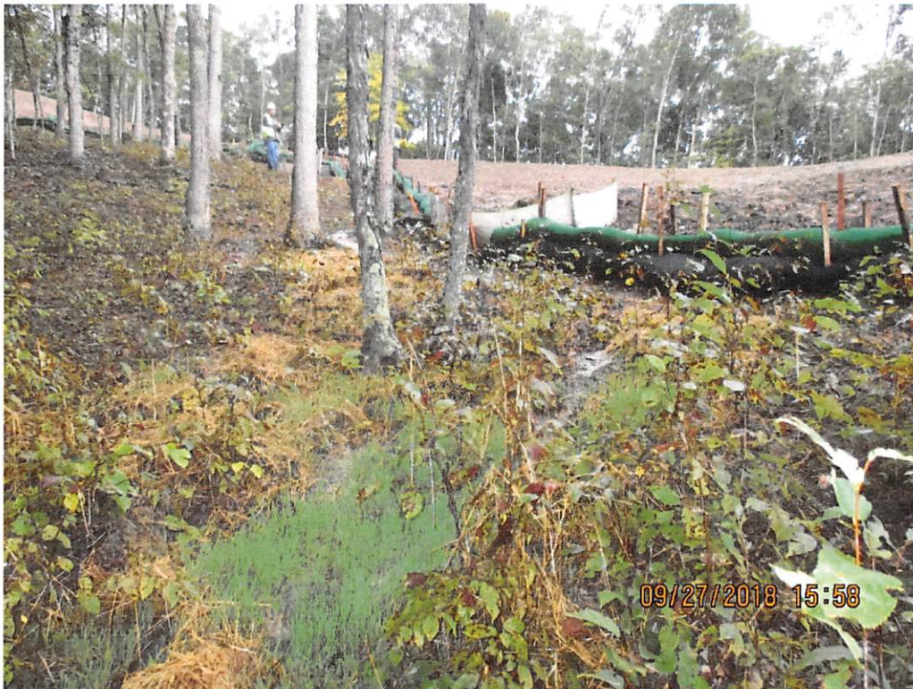
Areas near station number 9417+75 where water bar terminus being overwhelmed with sediment laden water.
