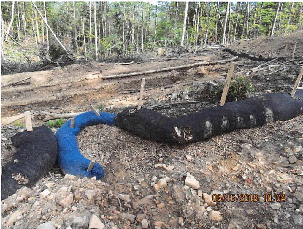
Photo 12: CFS needs maintenance near Bingham Road station 7450+00.
