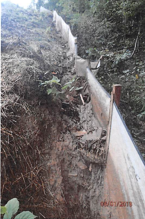
Concentrated flow being channeled along perimeter control trench due to improperly installed water bars in the Goose Run watershed.
