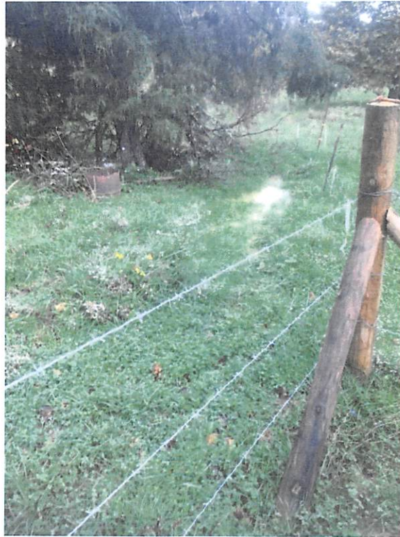
Sediment laden water infiltrating past LOD and seeping into wetland (W-22) and entering stream (S-Z3) near station number 9784+00.
