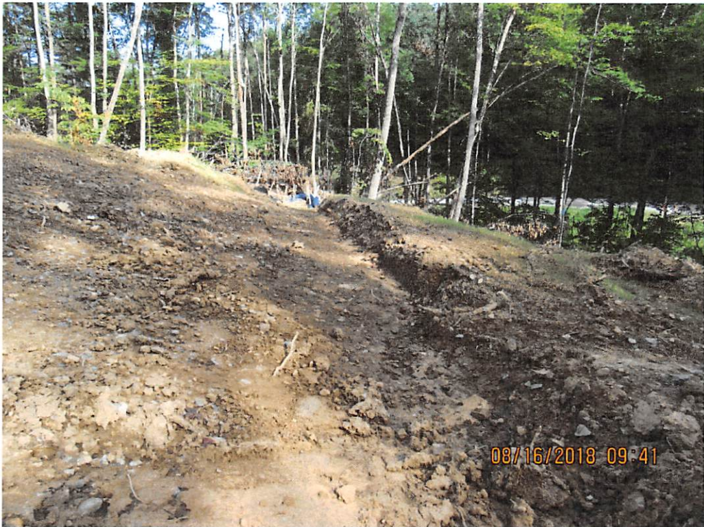
Photo 2: Western view of one of several incorrectly sloped water bars in Photo 1 off Bingham Road station 7450+00.
