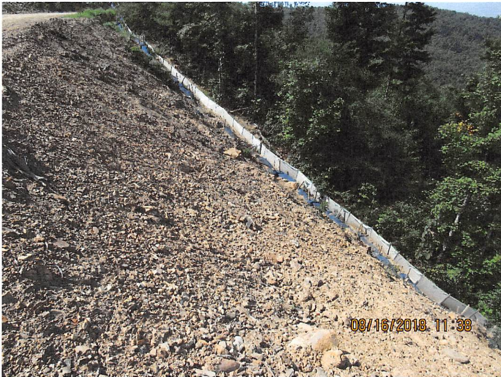
Photo 16: Southern view of Bamboo Road near Station 7158+00 without fill slope protection and temporary stabilization.
