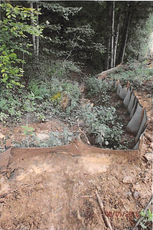
Perimeter control that has been overwhelmed due to concentrated flow from improperly installed water bars in the Goose Run watershed.
