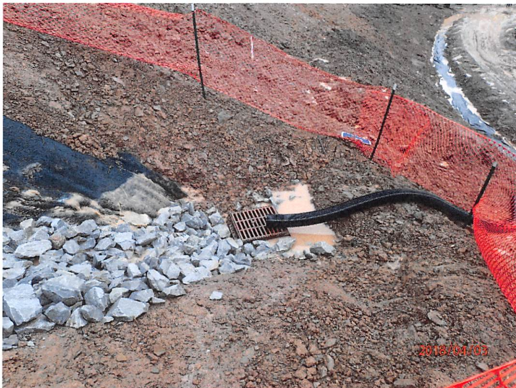
Unprotected drop inlet at Mobley Compressor Station.
