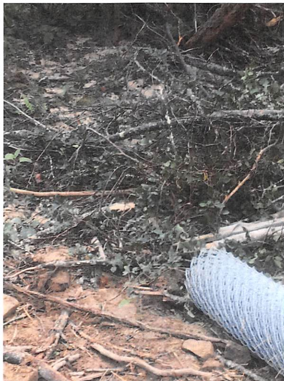
Close up of sediment that has been deposited past BMP.
