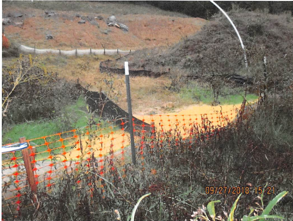
Lack of fill slope protection causing erosion and sediment laden water to accumulate and overwhelm BMP.
