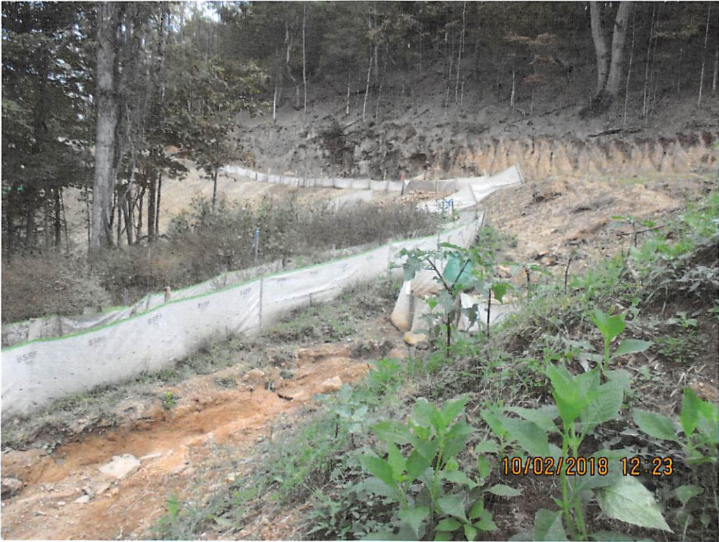
Lack of fill slope protection and channel stabilization enhancing erosion and causing BMP to be overwhelmed at station 9687.
