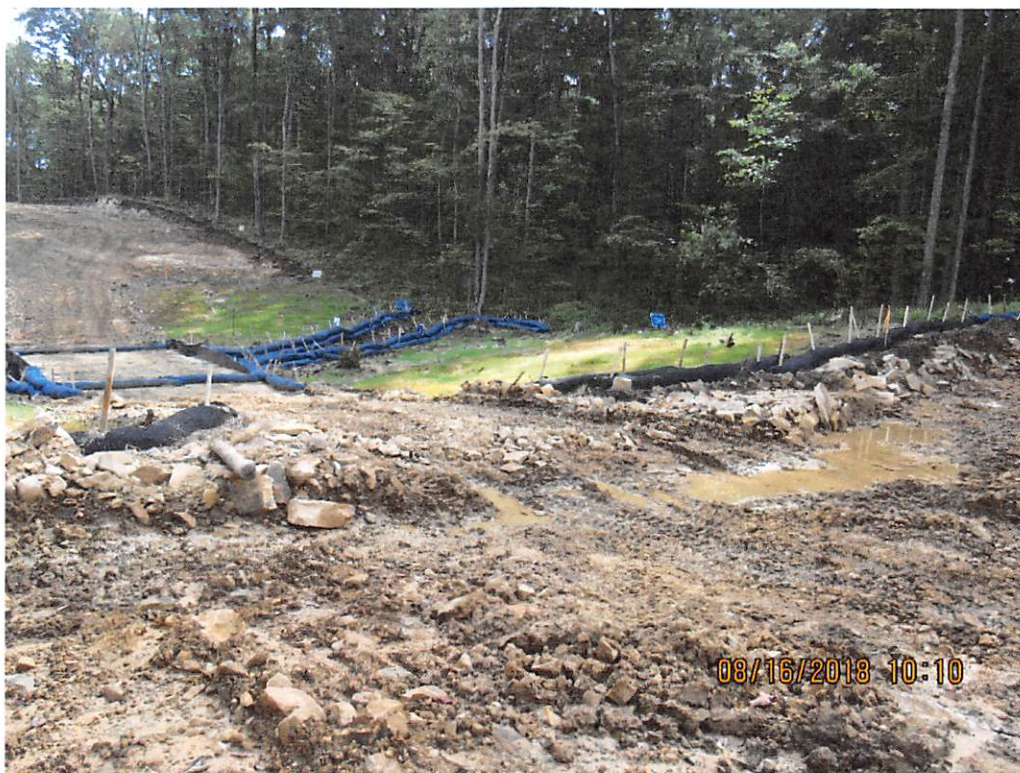
Photo 7: Middle section of water bar without outlet near Bingham Road station 7450+00.
