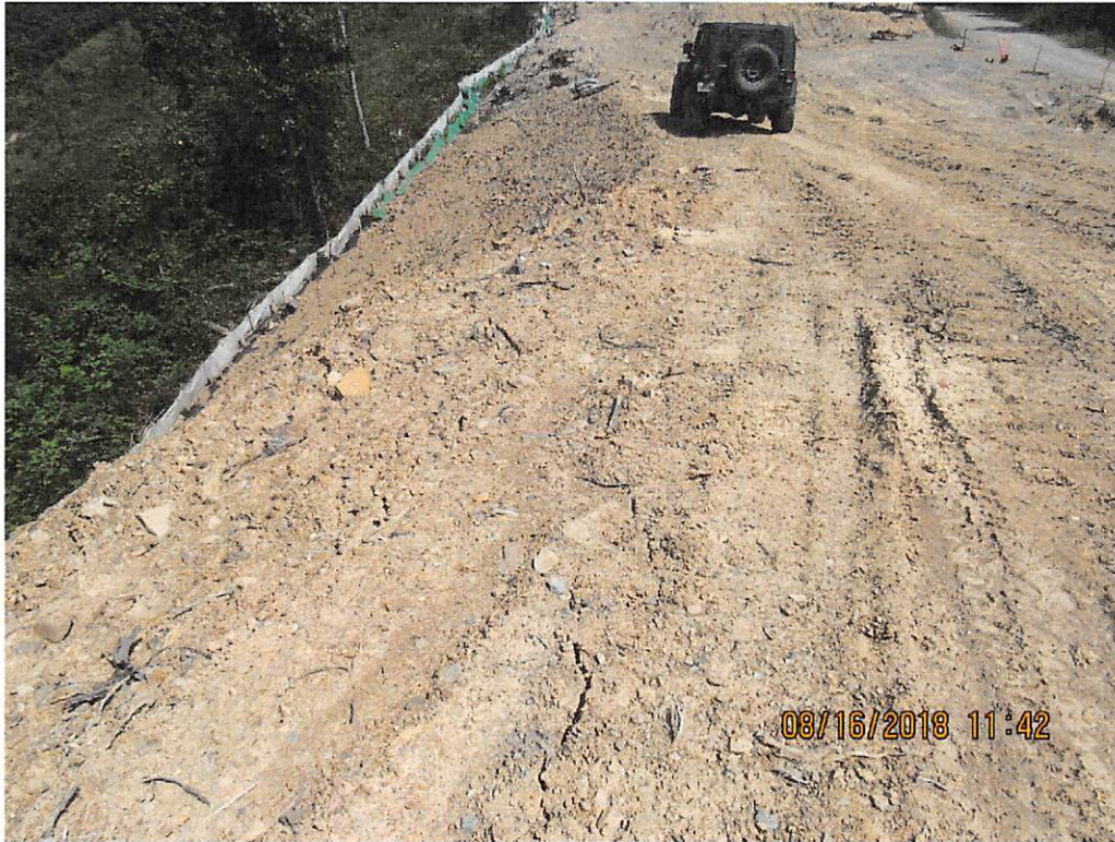
Photo 15: Northern view of Bamboo Road near Station 7158+00 without fill slope protection and temporary stabilization.
