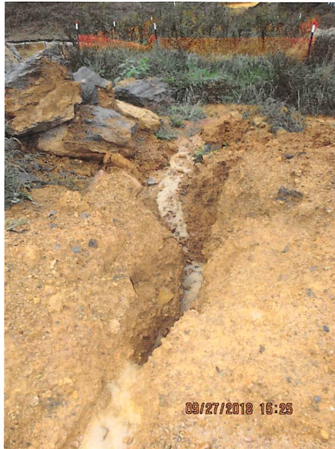
Water bar terminus leading to BMP. Erosion occurring due to channel not being stabilized.
