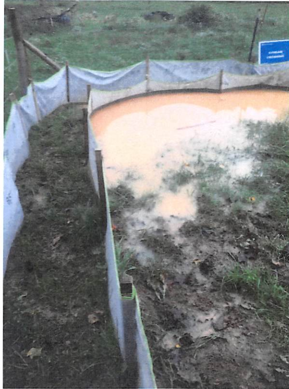
Area on south side of Ellison ridge road and ROW near station number 9784+00.
