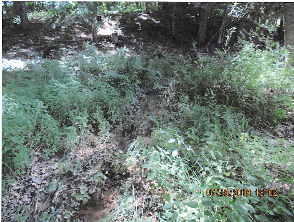
Photo 12: Terminus of sediment laden water leaving site from control failure near station 6785+50 (between MP 128.3 & 128.5)
