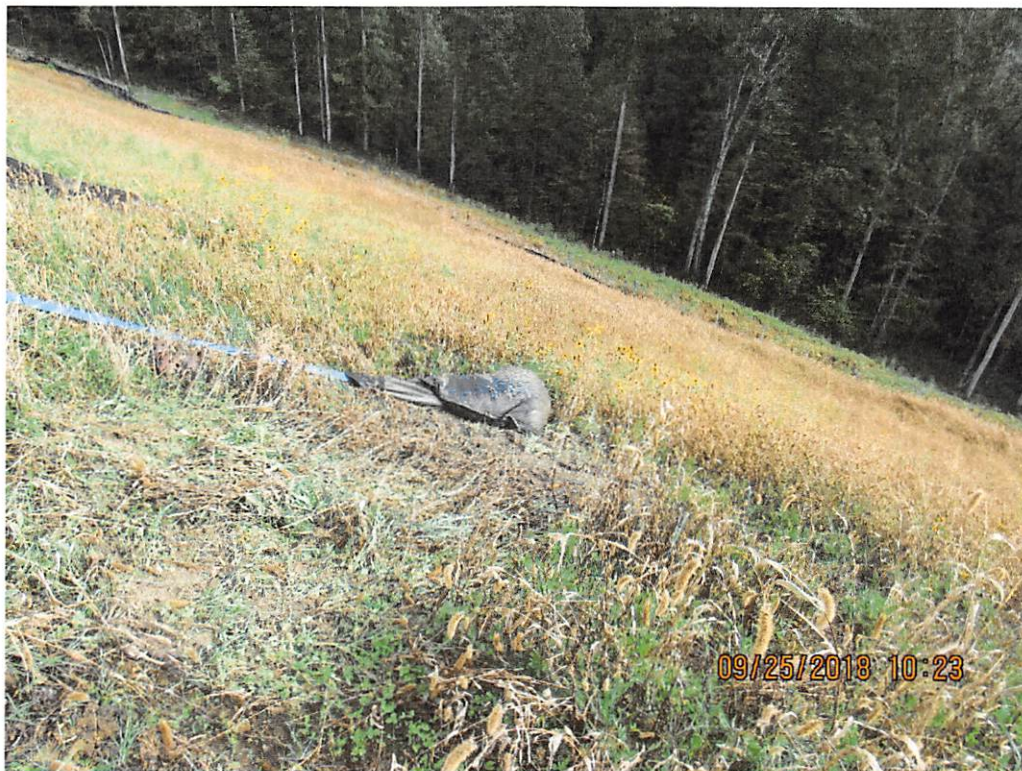
Photo 4: 1 of 3 improperly installed filter fabric bags still in use on north eastern side of site.
