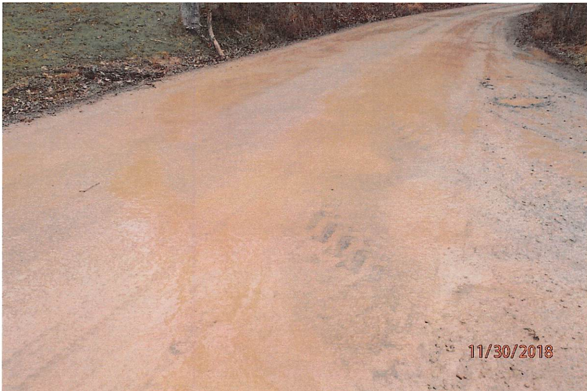
Access Road WV-HA - 29.04 off CR 50/5 showing the lack of an adequately stable construction entrance and the associated track out onto the public road.
