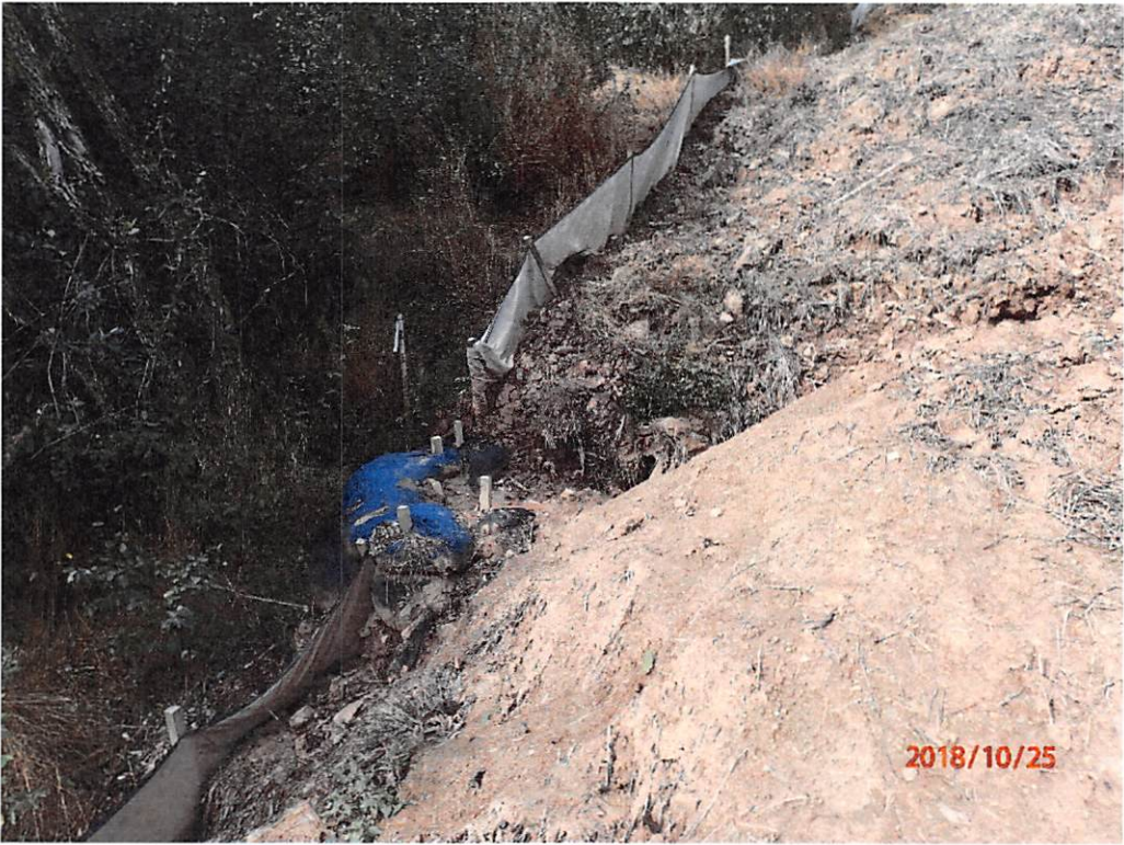
Overwhelmed sump near Sams Run.
