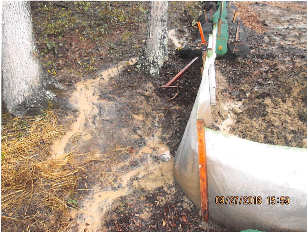
Areas near station number 9417+75 where water bar terminus being overwhelmed with sediment laden water.
