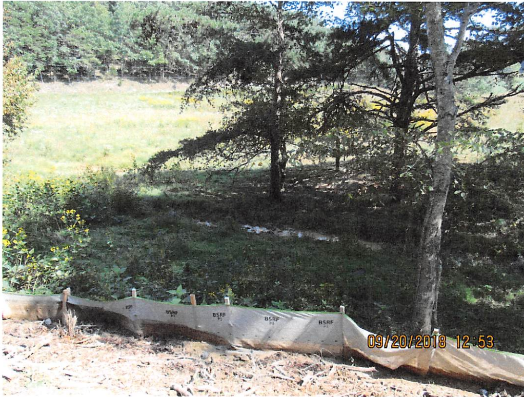
Photo 3: Sediment laden UNT of Painters Run down stream of control failure near station 10270+49
