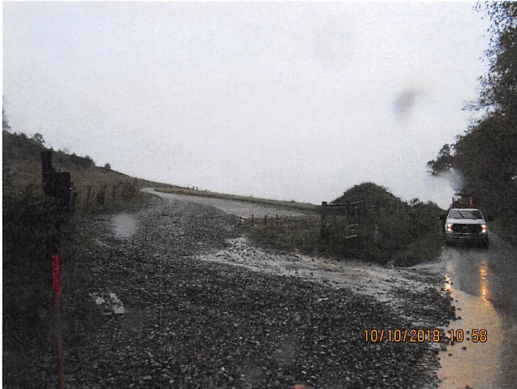
Photo 1: AR 210- sediment laden water leaving site.
