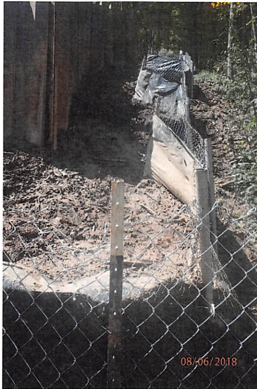
Sheet flow BMP adjacent to Rockcamp Run that is being utilized to treat concentrated flow from previously pictured unstable diversion that collects stormwater from water bars.
