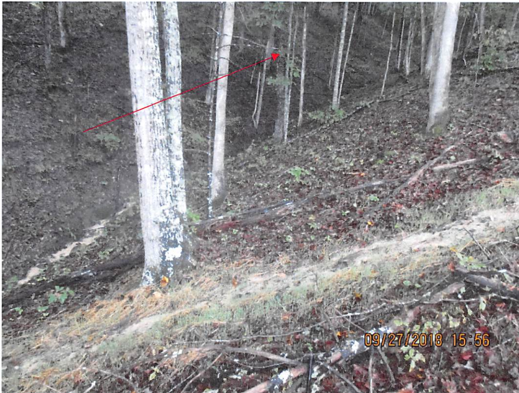
Sediment laden water being transported off ROW and past LOD into ephemeral streams near Station #9417+75. Red arrow depicts where ephemeral splits and goes upslope towards spring.
