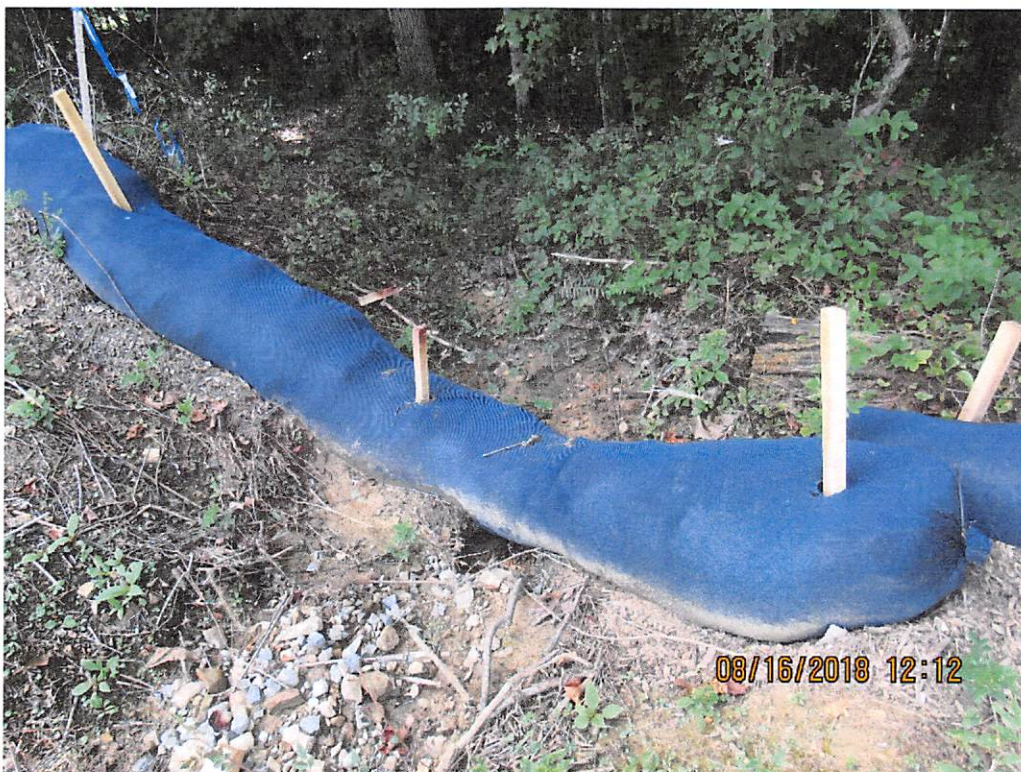
Photo 30: Perimeter controls failure downslope of SR culvert outlet allowing sediment laden water to leave site.
