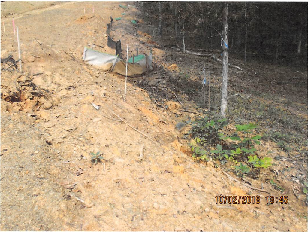
Waterbar outlet at station #9724+51 failing and off-site sediment deposits observed.
