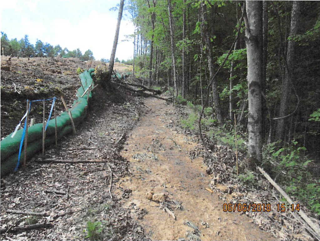
Photo 5: Scoured path from control failure at station 6812+58.
