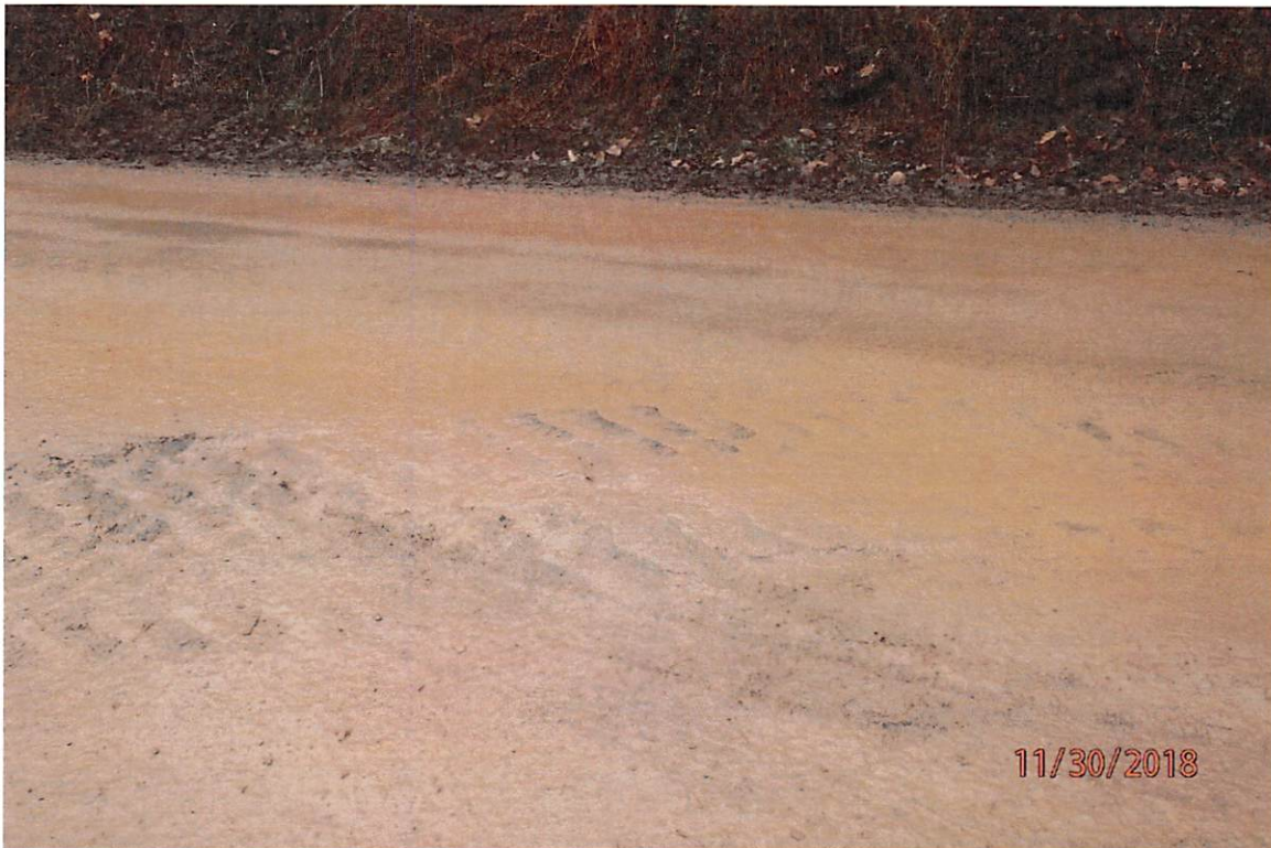
Access Road WV-HA - 29.5 off CR 50/5 showing the lack of an adequately stable construction entrance and the associated track out onto the public road.
