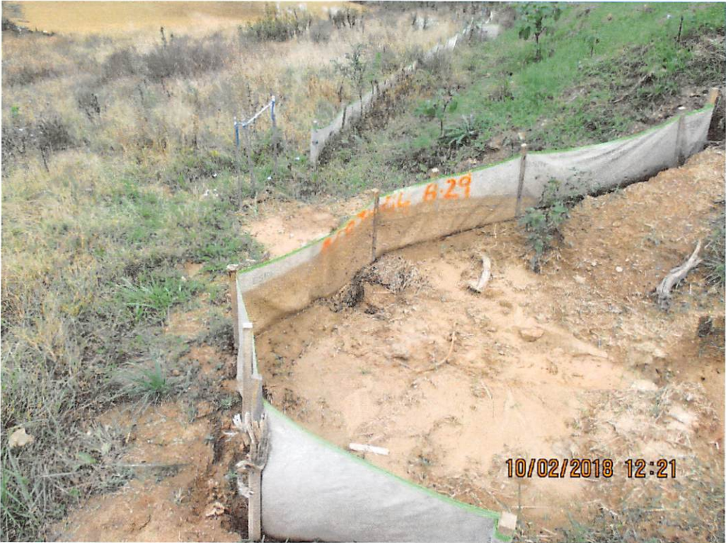
Off site sediment deposits past BMP near station number 9687.
