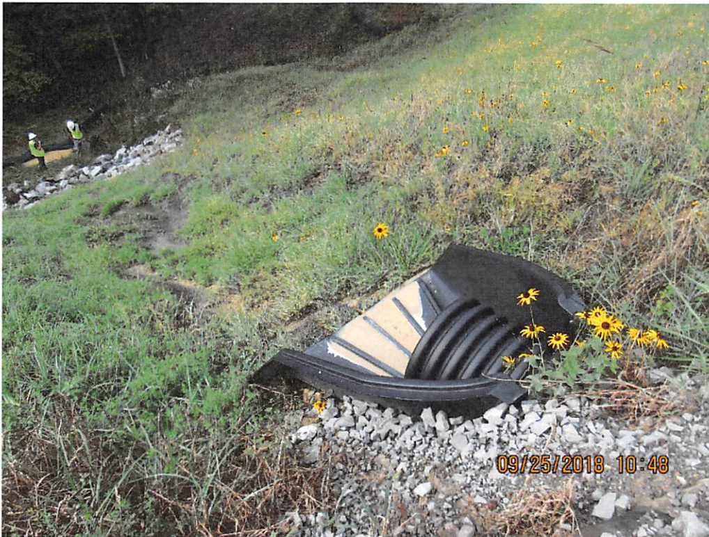
Photo 1: Station 550 outlet and sump at base of fill slope where perimeter controls failed allowing sediment laden water to leave site and create conditions not allowable in UNT of Little Kanawha.
