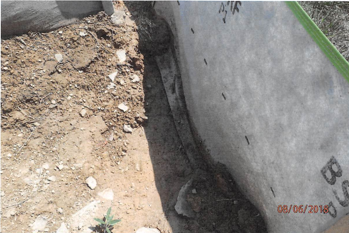
BMP in Seal Run watershed in need of maintenance that led to offsite sediment deposits.
