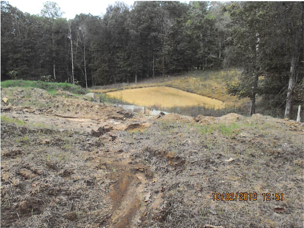
Gully erosion occurring near Station #9687 and flowing towards Pond (P-D2). BMP pictured was failing and off-site sediment deposits were present past the LOD.
