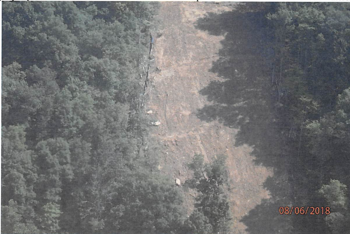
Improperly installed water bars and associated fill slope erosion in the Little Rockcamp Run watershed.
